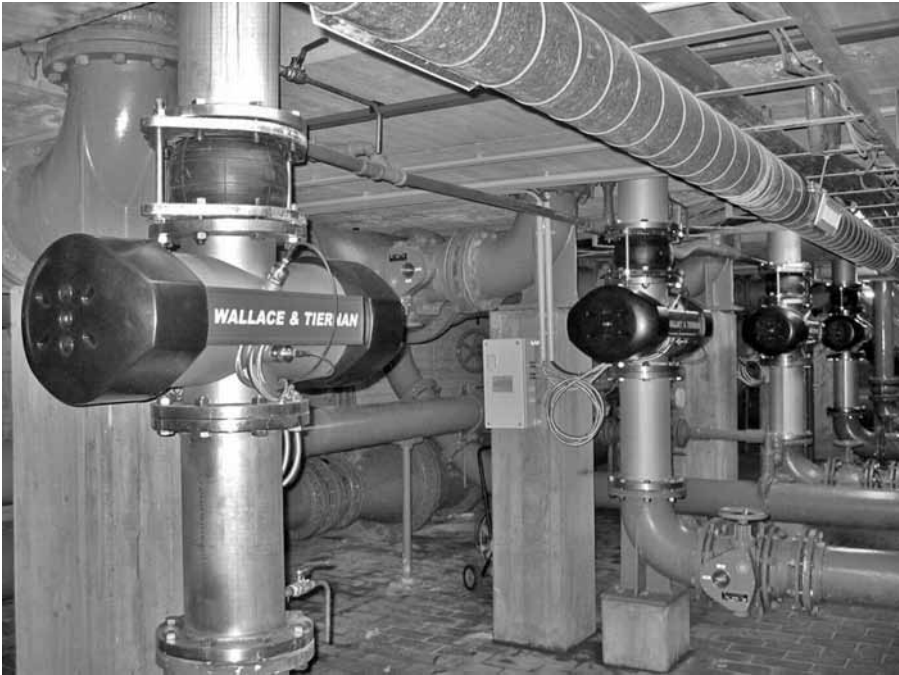
Figure 7.16 Ultraviolet disinfection installation. UV units are small and have very short radiation residence time. Courtesy Siemens press picture.
