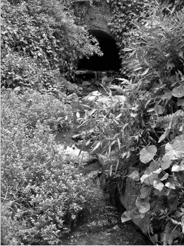
Figure 9.12 Daylighted and restored Strawberry Creek on the campus of University of California, Berkeley. Blocks from the removed culvert were used to stabilize the banks.
