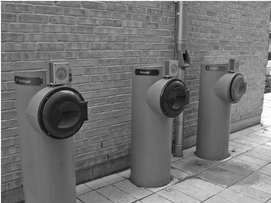
Figure 10.13 Solid waste disposal site in Hammarby Sjöstad in Stockholm, Sweden. Each disposal chute is connected to the underground system for handling different types of solid waste. Photo courtesy Malena Karlsson, GlashusEtt, Stockholm, Sweden.
