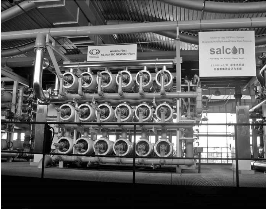
Figure 7.14 Installed reverse osmosis units in NEWater plant in Singapore. Photo V. Novotny.
