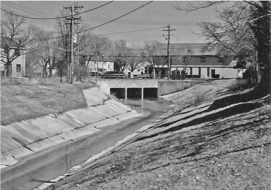
Figure 9.10 Fragmentation by culverts and concrete lining. Shallow channels with no pools are uninhabitable by aquatic biota, except by some attached growth slimes. Photo V. Novotny.
