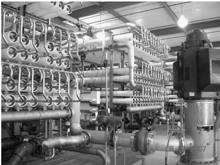
Figure 5.14 Reverse osmosis in the El Paso desalination plant (courtesy CDM).
