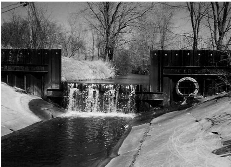
Figure 4.3 Stream lining with a drop structure was the third and fourth paradigm engineering solution to reduce erosivity of urban streams. Biota cannot develop in such channels and cannot pass the drop structure when migrating from downstream to upstream. Photo V. Novotny.
