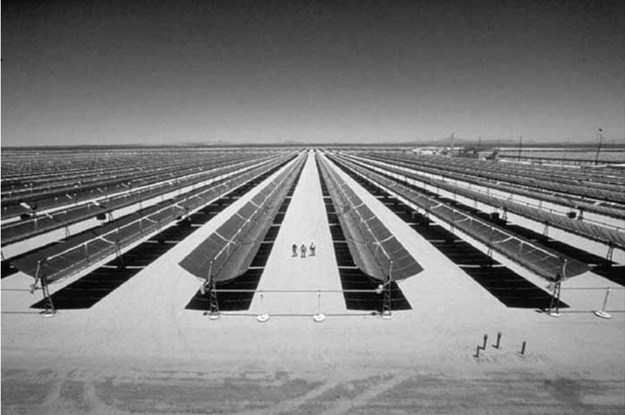
Figure 8.14 Trough mirror array of the solar panel in Kramer Junction, one of the largest concentrated solar energy farms in the U.S. Photo courtesy of Sandia National Laboratory.
