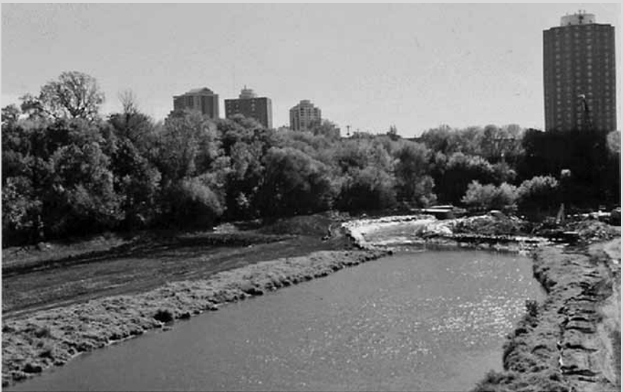
Figure 9.27 Dam removal, sediment capping, and stream bank armoring of the North Avenue impoundment in 1995. Photo V. Novotny.
