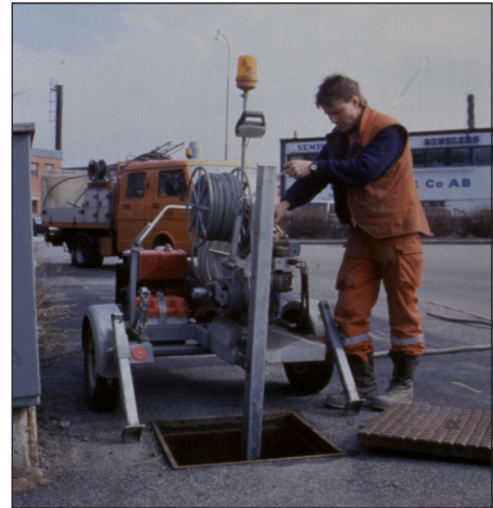
Fig. 11-13 Microprocessor-controlled winch for cable laying in ducts. (Photo, courtesy of Riteco AB)
