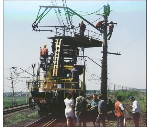
Fig. 11-26 Lashing optical fiber cable along a railroad. The cable is lashed to the neutral wire.
