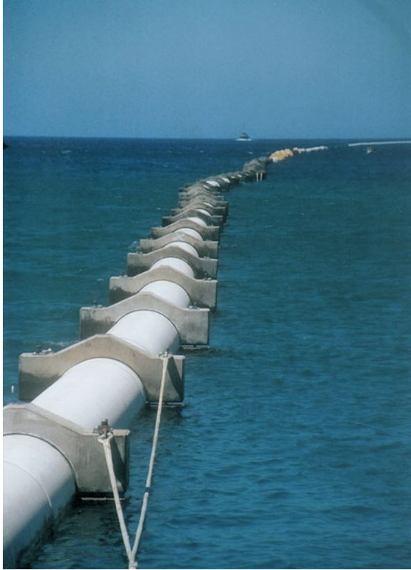
Fig. 11.3 Deep seawater intake pipes being laid out to sea for SWAC cooling at Kawaihae by Makai Ocean Engineering, Hawaii (Credit: Makai Ocean Engineering)
