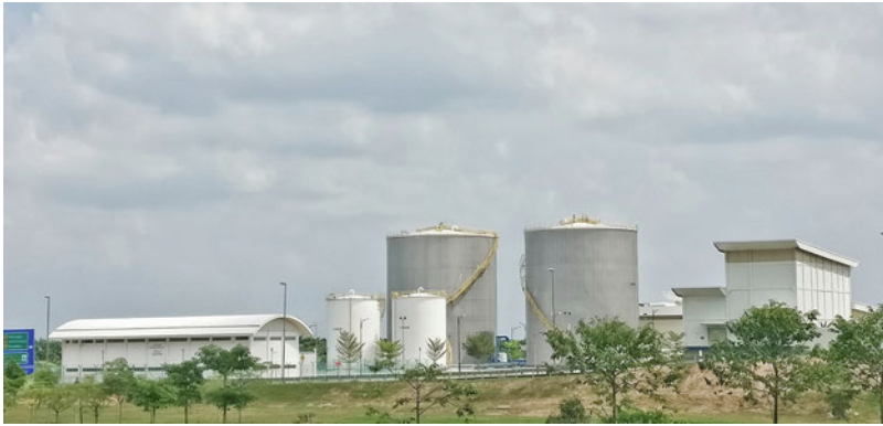
Fig. 11.5 District cooling plant at Kuala Lumpur Airport KLIA (Source: Danny Tam Hong Khai)
