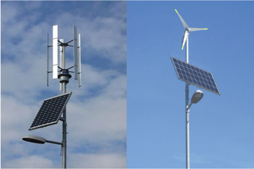
Fig. 4.4 Photos of the off-grid power system built in the premises of the VŠB-TUO; the usage of two hybrid power sources
