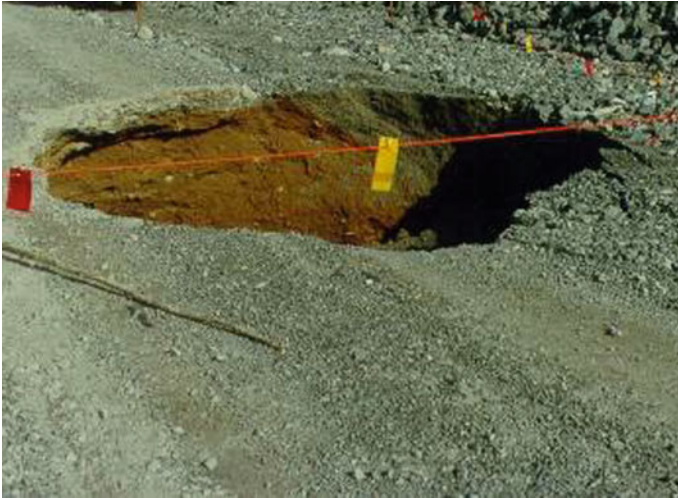
Fig. 5.10 Sinkhole in embankment surface caused by poor CQA on filter zone
