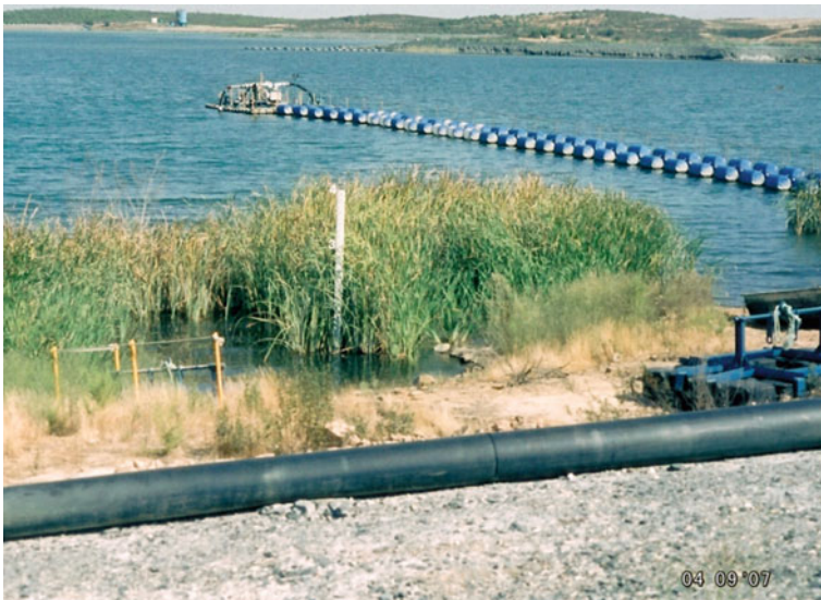
Fig. 6.50 Floating barge pump at IRCL, Portugal
