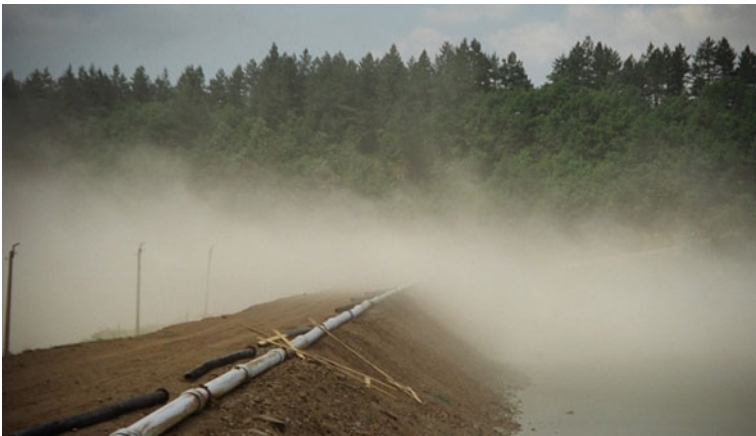
Fig. 6.44 Resulting dust issues
