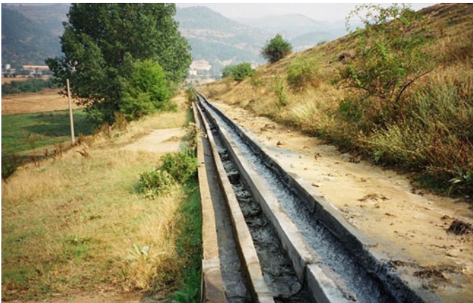
Fig. 6.21 Concrete tailings launder with multiple channels
