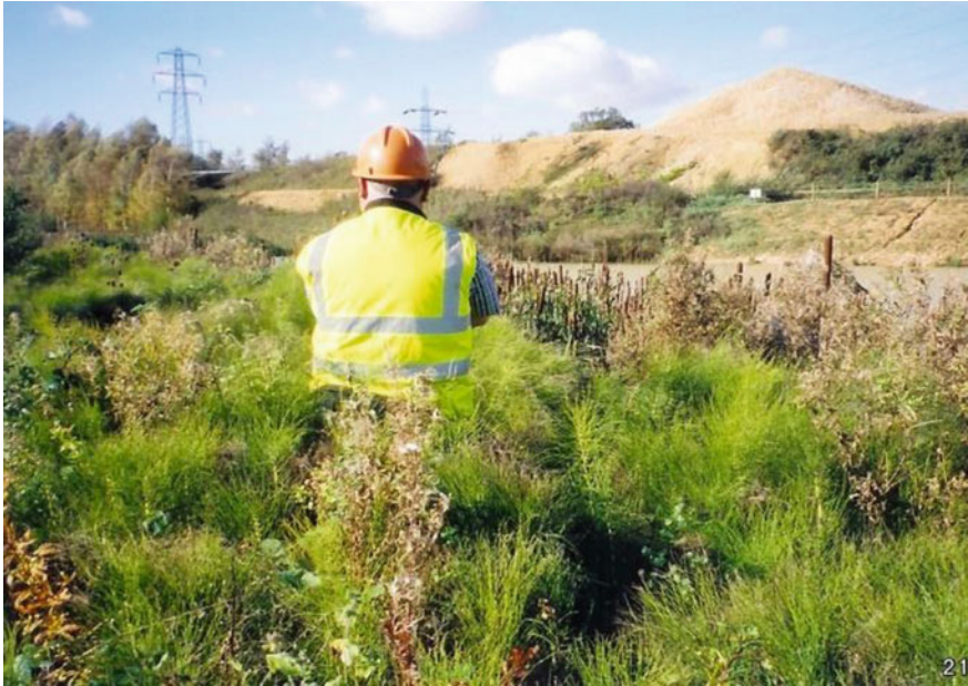
Fig. 7.10 Crest of embankment obscured by vegetation
