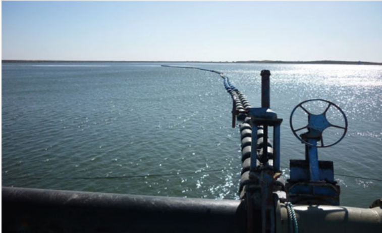
Fig. 6.18 Floating tailings delivery pipeline
