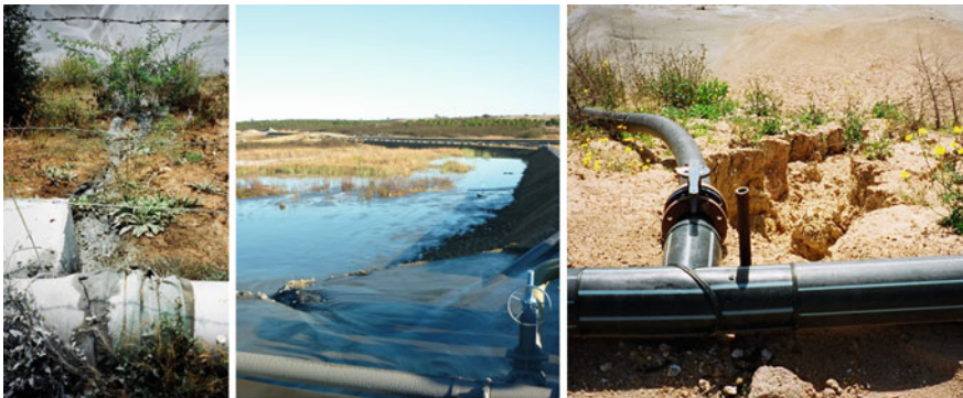
Fig. 7.13 Poor maintenance leading to uncontrolled discharges
