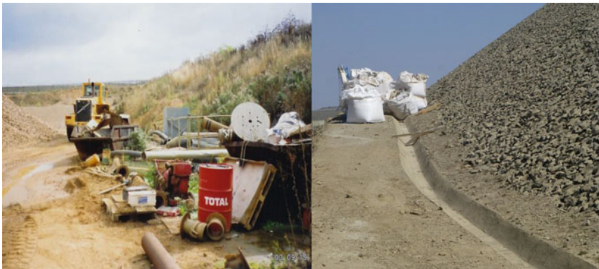
Fig. 7.11 Storage of materials against embankment toe
