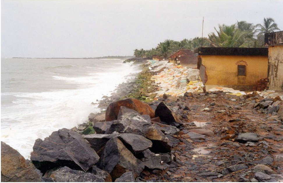
Shoreline Changes, Figure 7 Fury of the monsoon waves slashing the coastline with intensive erosion. Surf zone between the wave break and shoreline is well developed. Seawall is built as a protective feature (Photo: K.S. Jayappa).
