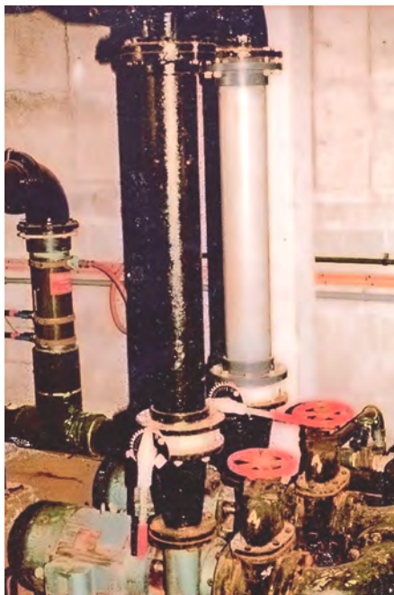
Figure 1.3 An example of metal corrosion and replacement of a length of corroded metal pipe with a plastic alternative
