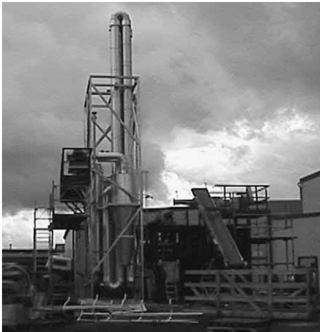
FIGURE 14.9 Acetylation pilot plant being assembled in Kvarnatorp, Sweden.
