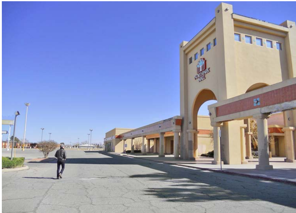
Figure 5.2: Northpark Mall, El Paso, Texas. Existing conditions in 2010. The sprawl experiment eventually led to spectacular commercial failures like this one, all over North America.
