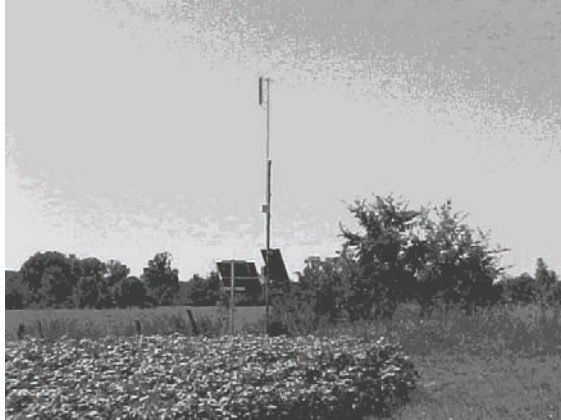
Figure 2. Picture of repeater station with sectorial antenna at top, square panel antenna communicating to base station in the middle of the picture and solar panels for power at the bottom of the tower
