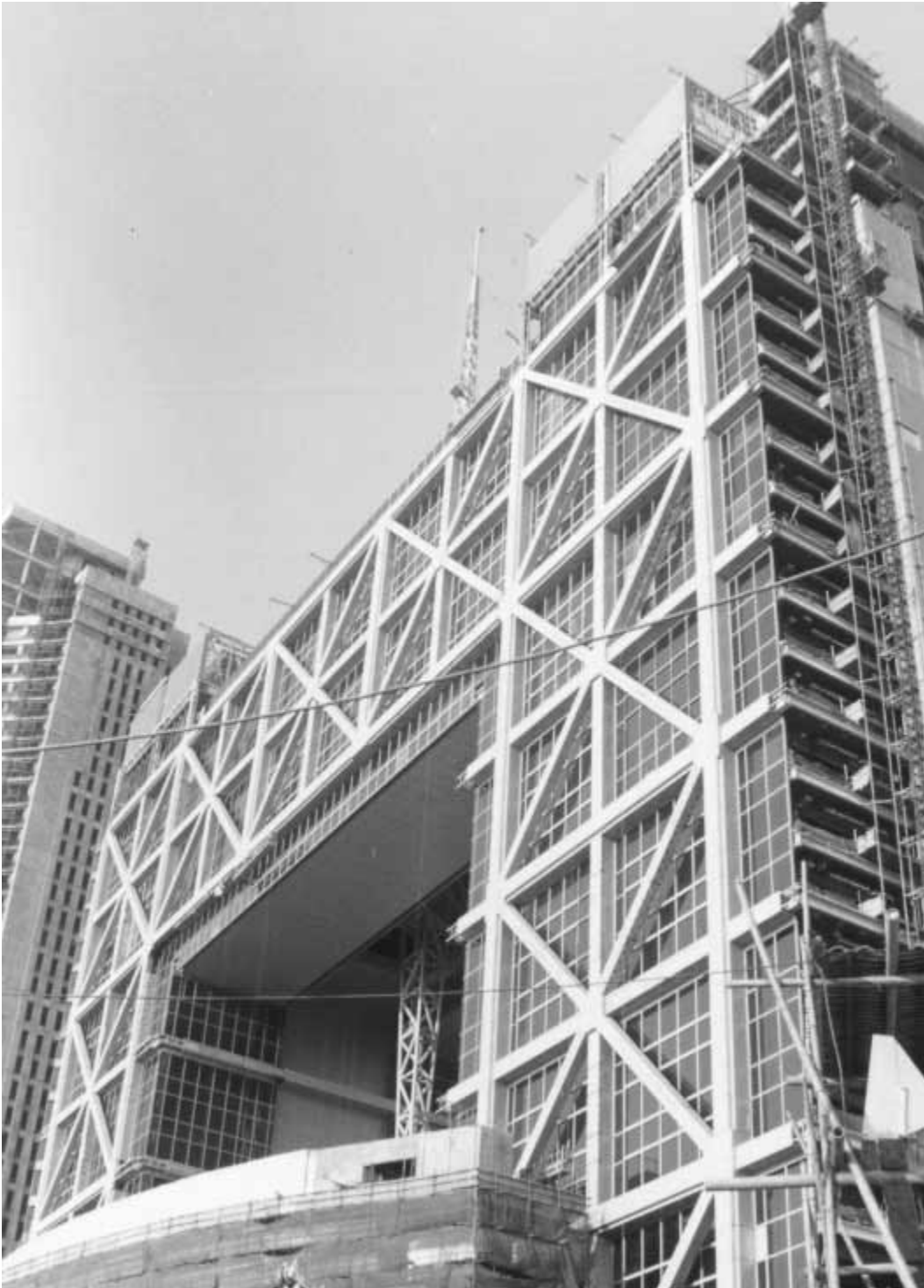
58 The Shanghai Securities Exchange Building, Pudong, Shanghai, by WZMH and the Shanghai Institute of Architectural Design and Research, ca. 1995.
