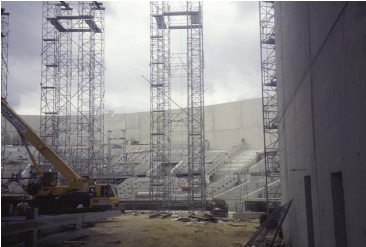
Assembly of temporary structure to support roof until masts and cables were in place
