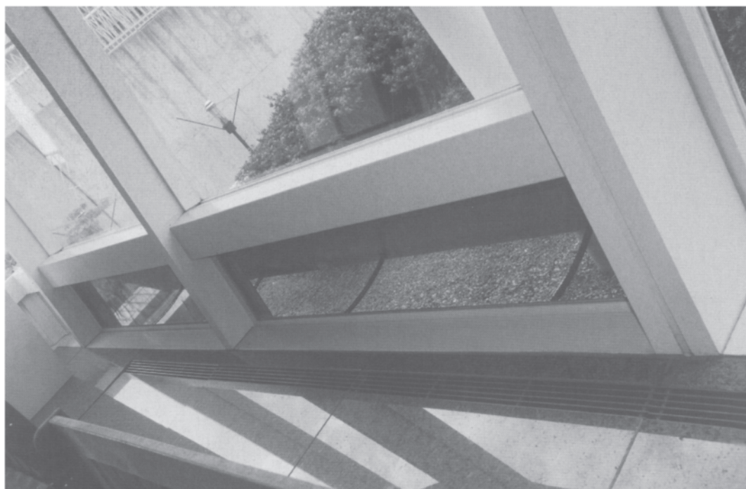
12.6 Interior view of a ventilation opening at the bottom of the atrium glazing.
