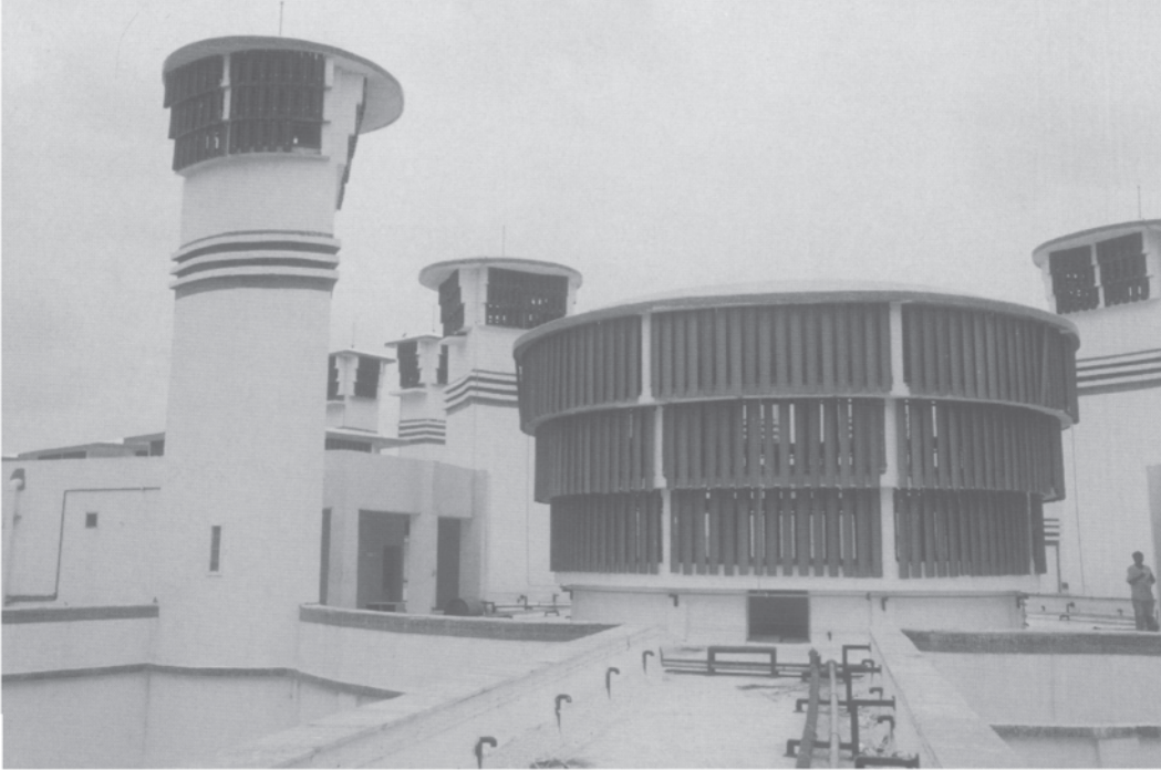
17.8 Circular air inlet tower to the Core Building flanked by some of its taller air-extract towers.
