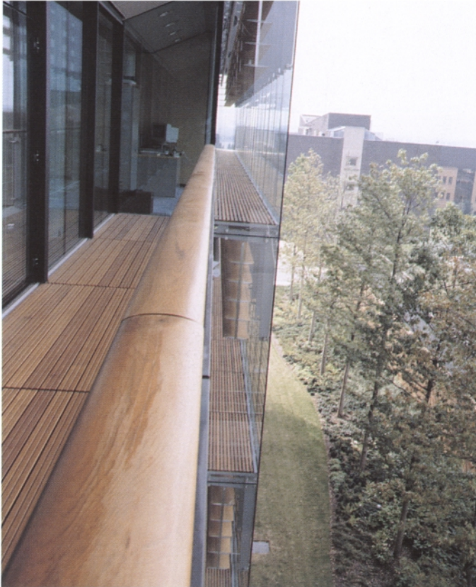
Plate 28 Glaxo-Wellcome Headquarters, London—walk-in cavity, looking south from the Board Room balcony on the second floor.
