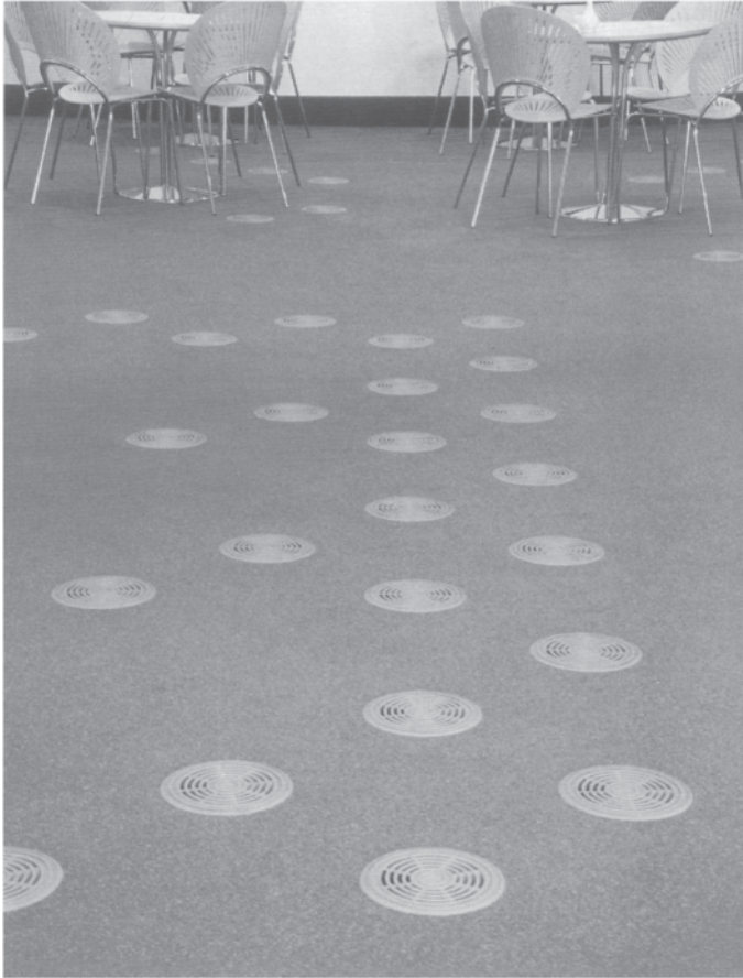
9.9 The Scottish Office, Edinburgh— air supply diffusers on the dining room floor.
