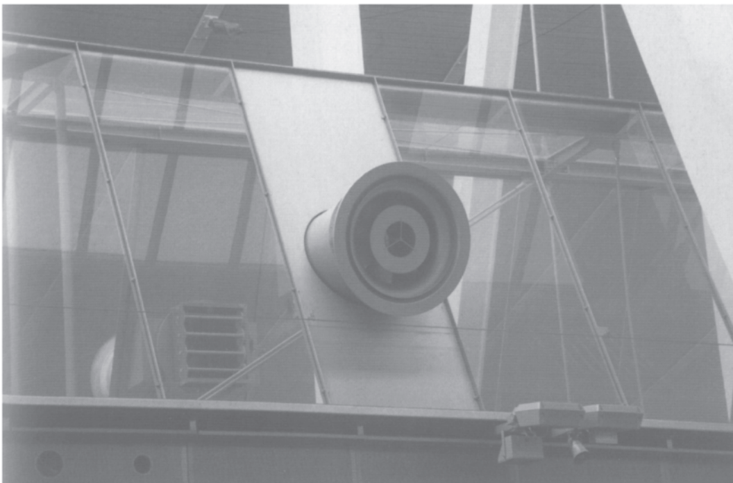
11.5 Close up of one of the warm air nozzles, with the control dampers of the one on the opposite side of the duct visible through the glass sides.
