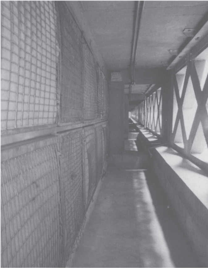
13.9 Filter bank between the fresh air inlet from the atrium (right) and the fan room (left, on the other side of the filters).
