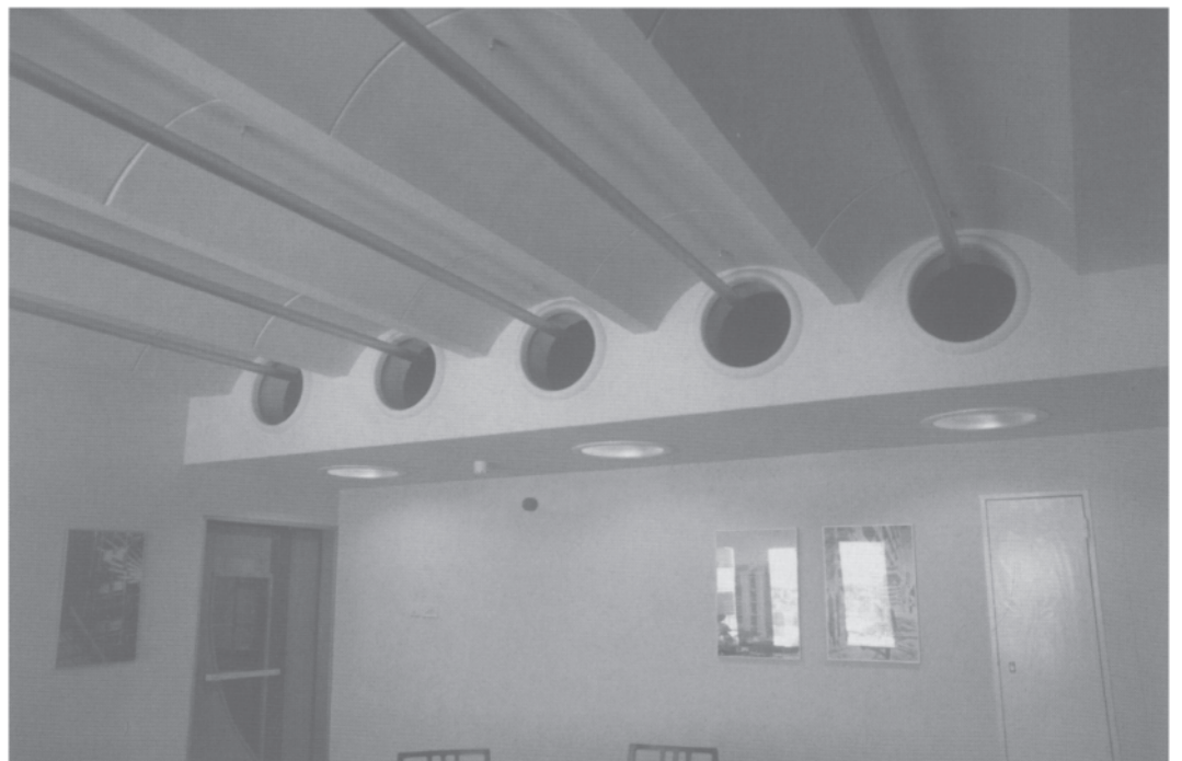
13.12 Circular exhaust air ports in the office areas.
