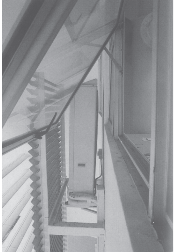
4.14 Condenser units adjacent to the opening windows of a naturally ventilated classroom, and immediately under the roof overhang.
