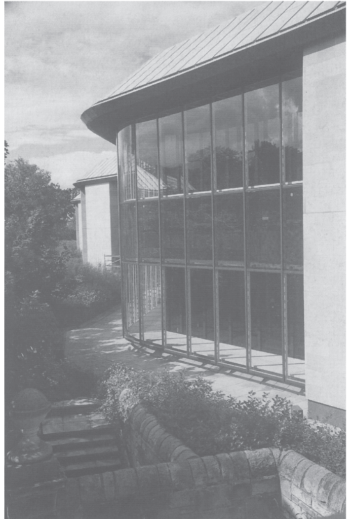
3.17 Tanfield House —double façade. Note the grille at the bottom to allow air movement, and the tinted band of glazing at mid-height, which obscures the air-handling units located there.
