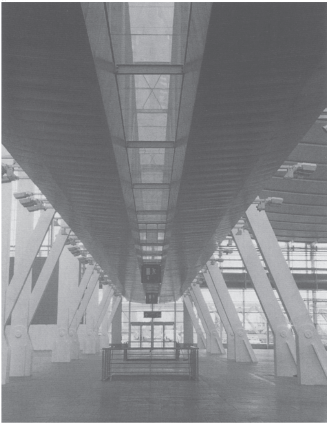
11.6 Underside of the transverse duct showing where the cool air is supplied.
