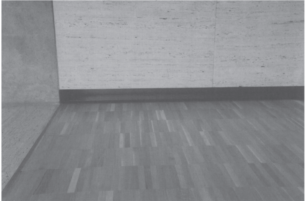
3.2 Kimbell Art Museum— close up of the floor-level linear air supply grille to an exhibition space.
