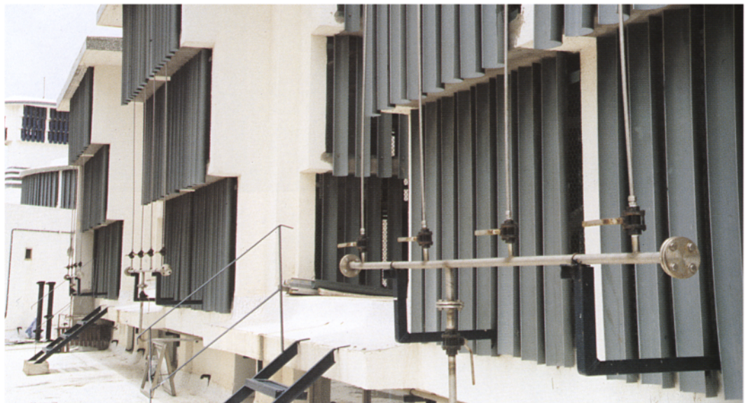
Plate 30 Torrent Research Centre, Ahmedabad—close up of the external pipework of the micronisers beside the air intakes to one of the Laboratory Buildings. Note also the vertical half-pipe arrangement designed to reduce penetration of sun and sand (plastic piping has been used pending the delivery of the intended green ceramic pipe).
