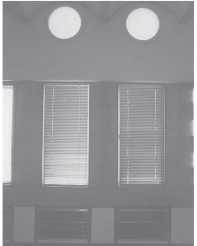
13.11 Air supply grilles under the perimeter windows. The grille on the left incorporates a small electric heater.
