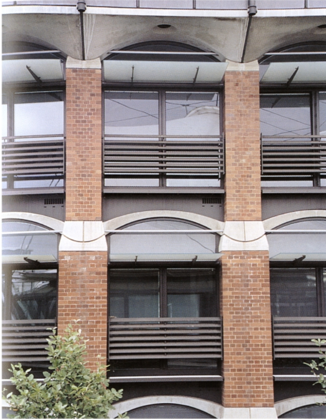
Plate 16 Inland Revenue Offices, Nottingham —typical section of the façade showing the balustrade and light-shelves with full-height glazing behind. Note also the curved shape of the ends of the ceiling panels and the small fresh air inlet grilles.
