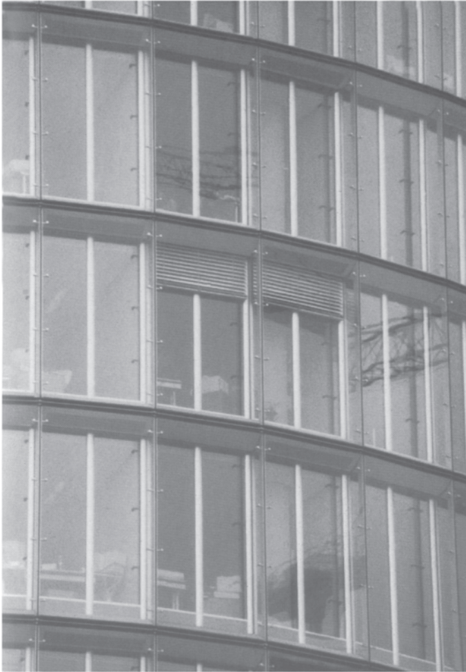
15.8 Close up of a section of the façade. Note the fish mouths and alternating pattern of perforated and non-perforated aluminium sheets at the tops of the glazed panels.
