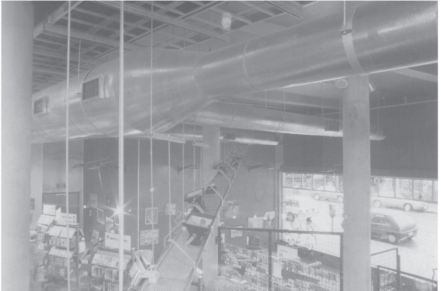
3.27 Palmerston North Public Library —air ducts and cable/lighting trays traversing one of the refurbished spaces (Sound and Vision Department).
