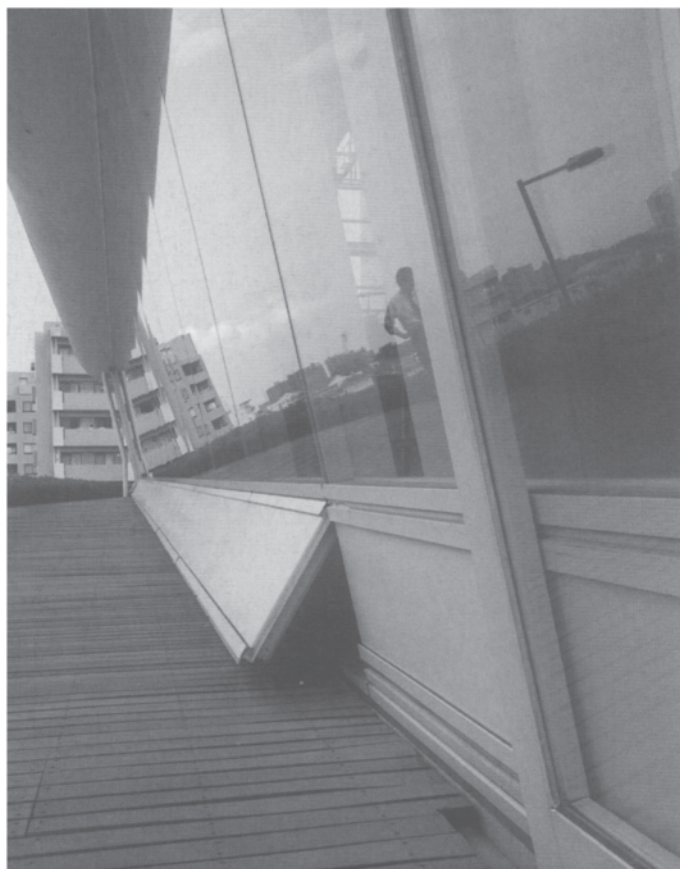
12.5 Exterior view of a ventilation opening at the bottom of the atrium glazing.
