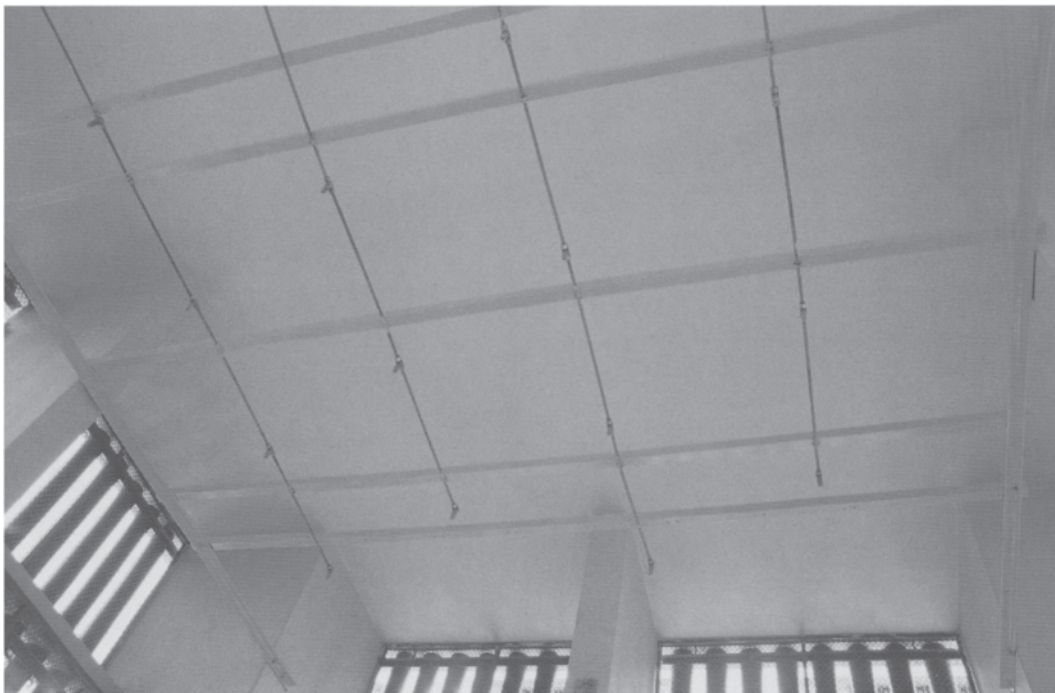
17.9 Typical microniser nozzle array supported on a frame inside one of the air intake towers. Note the absence of any louvres other than the half round pipes.
