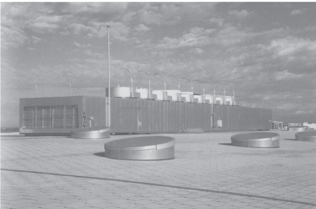
7.13 Skylights. The row on top of the metal-clad structure is above the atrium; the others are placed above the structural columns.
