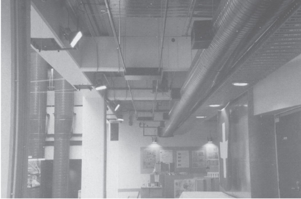
3.25 Wellington Schools of Architecture and Design—layering of the services. Note the fire sprinkler pipes, hot water heating pipes, air supply ducts and cable trays.
