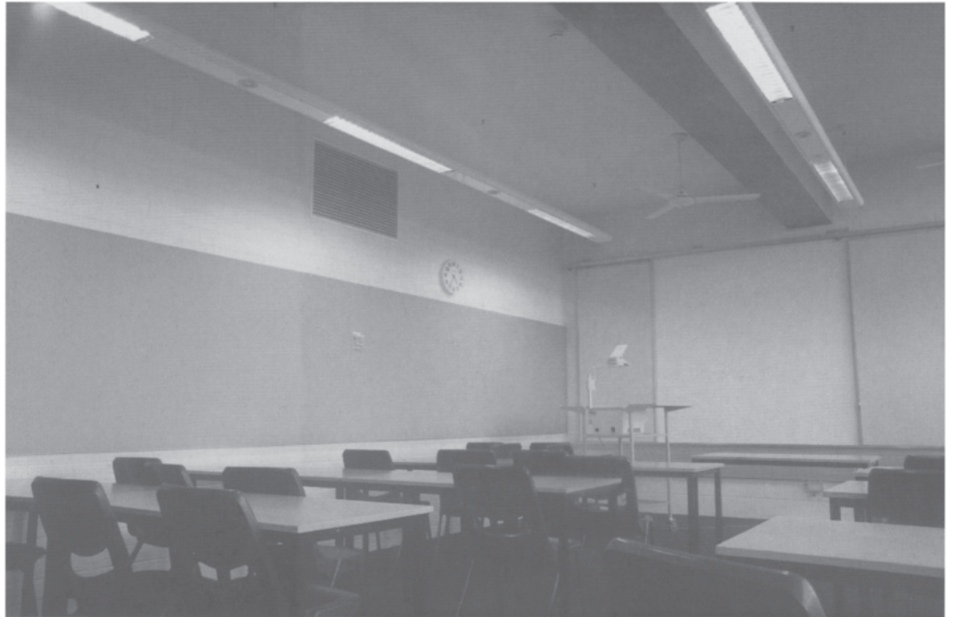
14.5 Typical classroom with an air-extract grille at a high level on an inner wall. Note the concrete block partition wall, exposed concrete ceiling and ceiling fan.
