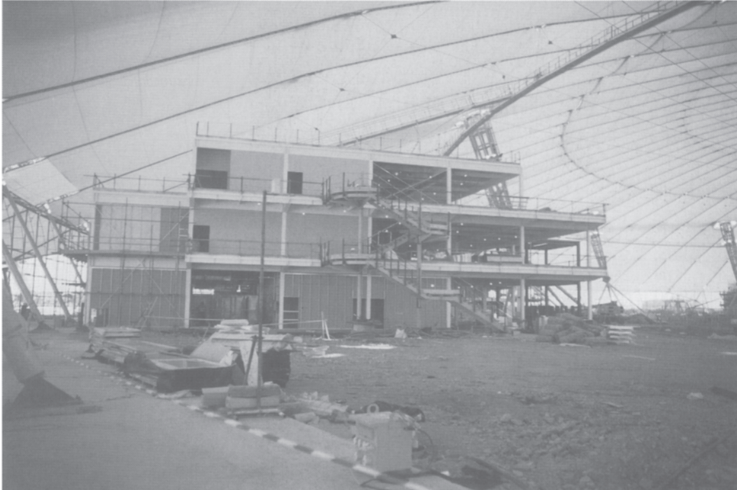
19.9 Millennium Dome, London —one of the six core services buildings at the inner edge of the Dome, when under construction in August 1998.
