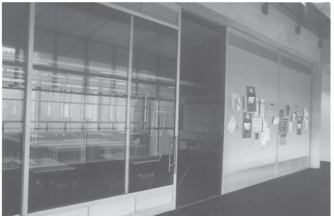
14.10 Sliding door/partition between the studio and corridor with fixed cross-ventilation louvres top and bottom.
