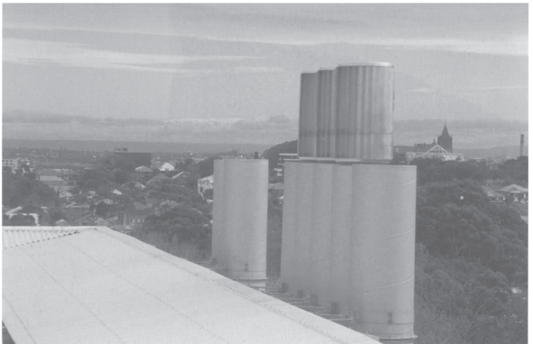
14.6 Upper section of a set of ventilation chimneys, some cowl-less as a result of hailstorm (note tarpaulins covering damaged suburban house roofs in the background).
