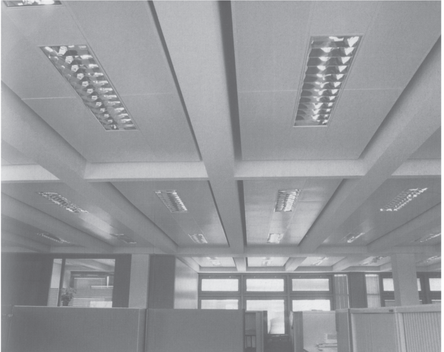
9.8 Typical office ceiling indicating the 'floating' suspended ceiling panels. Note the gap between the edge of the panel and the bottom of the concrete double-T units to allow for air circulation.
