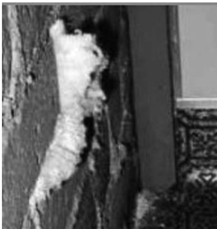
Crystallized efflorescence in a masonry wall.
