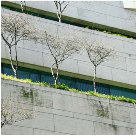
Green stains indicate moisture from the planters. Canadian Embassy, Washington, D.C., 1989.
