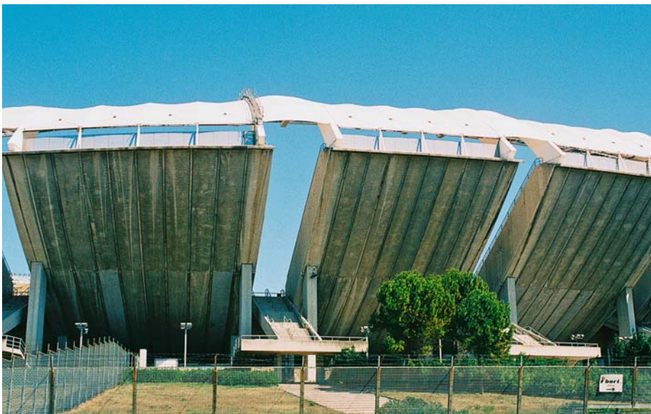
The San Nicola Stadium in Bari in the South of Italy, 1990, shows color differentiation across the concrete surface. Variation in the absorption of forms or inconsistent application of the form release agent can cause this type of discoloration.
