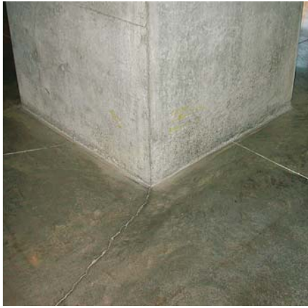
Cracks in the floor slab around an interior column oppose the anticipated crack direction. Cracking can be caused by improper isolation-joint design that does not provide relief at reentrant corners.
