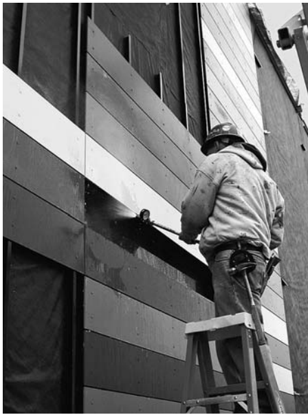
Field water test of cement fiber panel and window system transition. Gary Corner Youth Center, Chicago, 2006.
