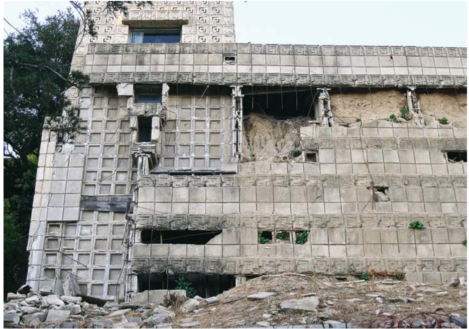
The Ennis-Brown House, Los Angeles, 1924. Exterior concrete block retaining walls crumbled after an earthquake and subsequent mud slides.
