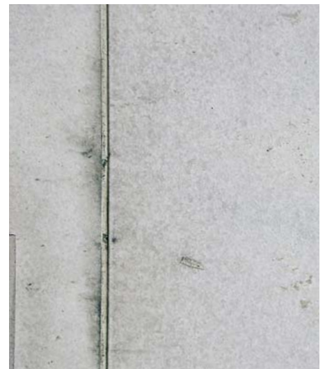
Stone replacement is the only method for removing the picture-frame effect of sealant joint stains.
