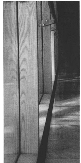
3.10 Detail of the air inlet slot at the sill of the great window
