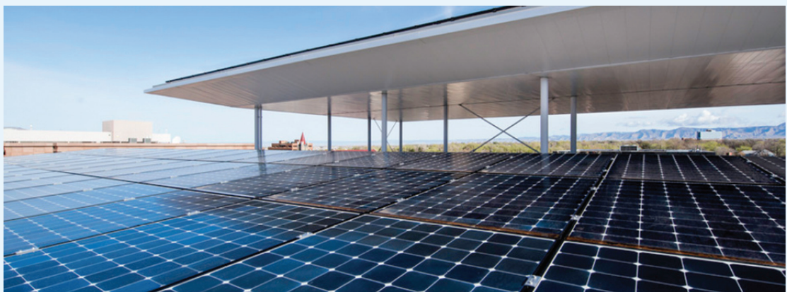
Figure 2-13 Rooftop PV array Photography by Kevin G. Reeves; Courtesy of DLR Group
