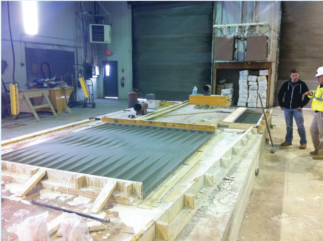
Figure 6-12 Photograph of a custom formliner at precast plant, RW Sidley in Thompson, OH Image courtesy of LMN Architects
