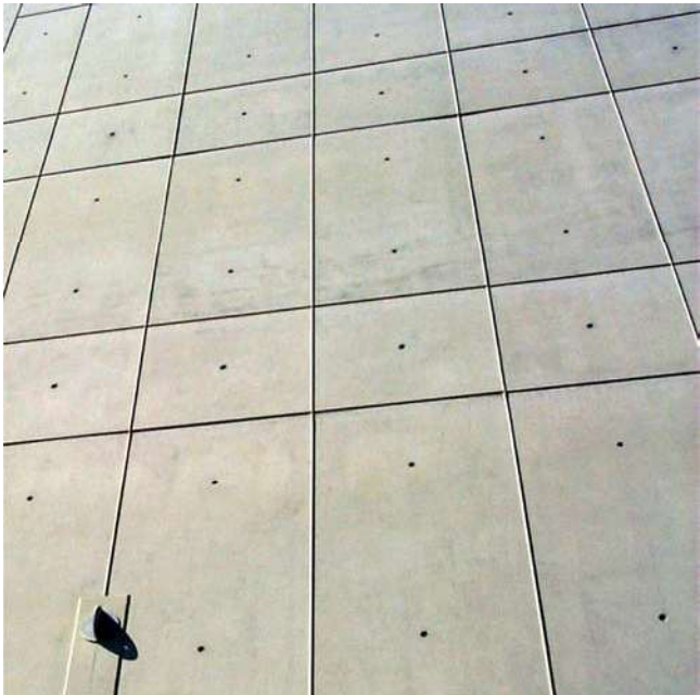
Fig. A.13—Outward reveals at the Amgen Building 29, Thousand Oaks, CA (Morley Construction, Santa Monica, CA).
