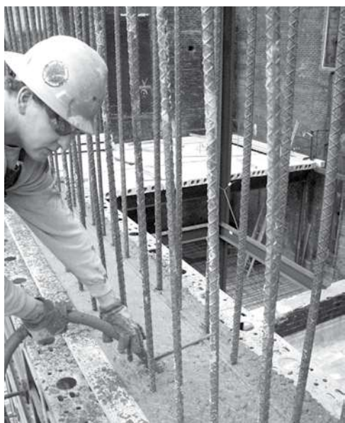
Fig. 8.2.1—Proper vibration of architectural concrete is vital to a successful and consistent product.
