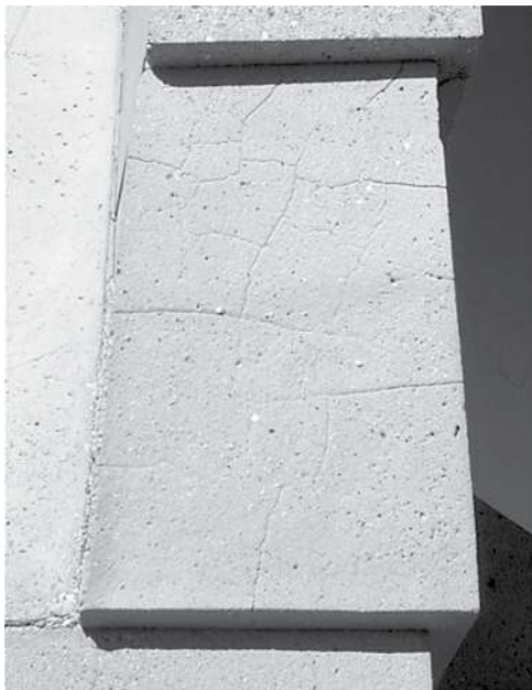
Fig. 5.10.2—Map cracking due to thermal shock; sandblasting emphasizes the cracks.
