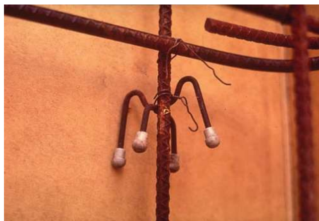
Fig. 6.3—Improperly installed reinforcing steel chair.
