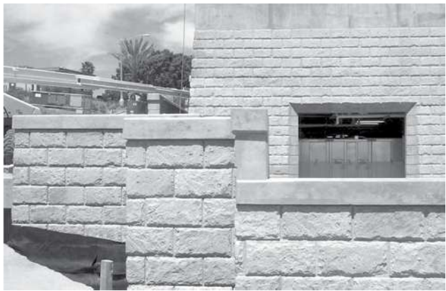
Fig. 5.6.2—Elastomeric form liner used to create a block pattern finish at the University of San Diego Science Center, CA.
