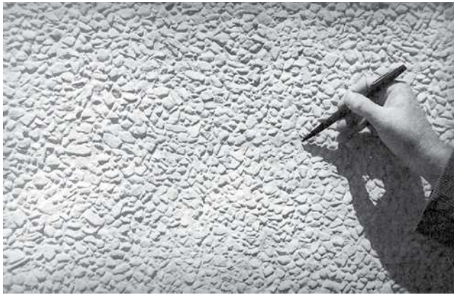
Fig. 7.2.2—A gap-graded, cast-in-place concrete mixture after heavy sandblasting. Note the preponderance of one-size material.
