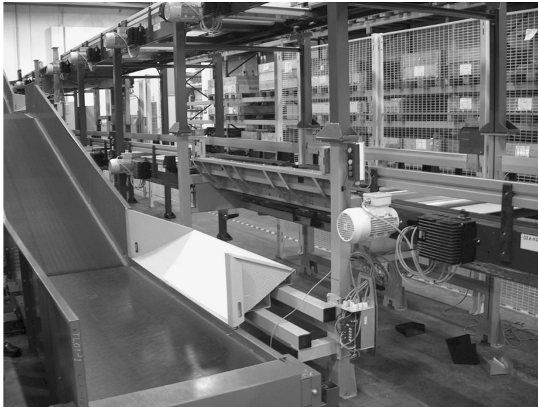
Figure 3.16 A discharger element that can tilt the tote, so bags slide onto the conveyor belt
