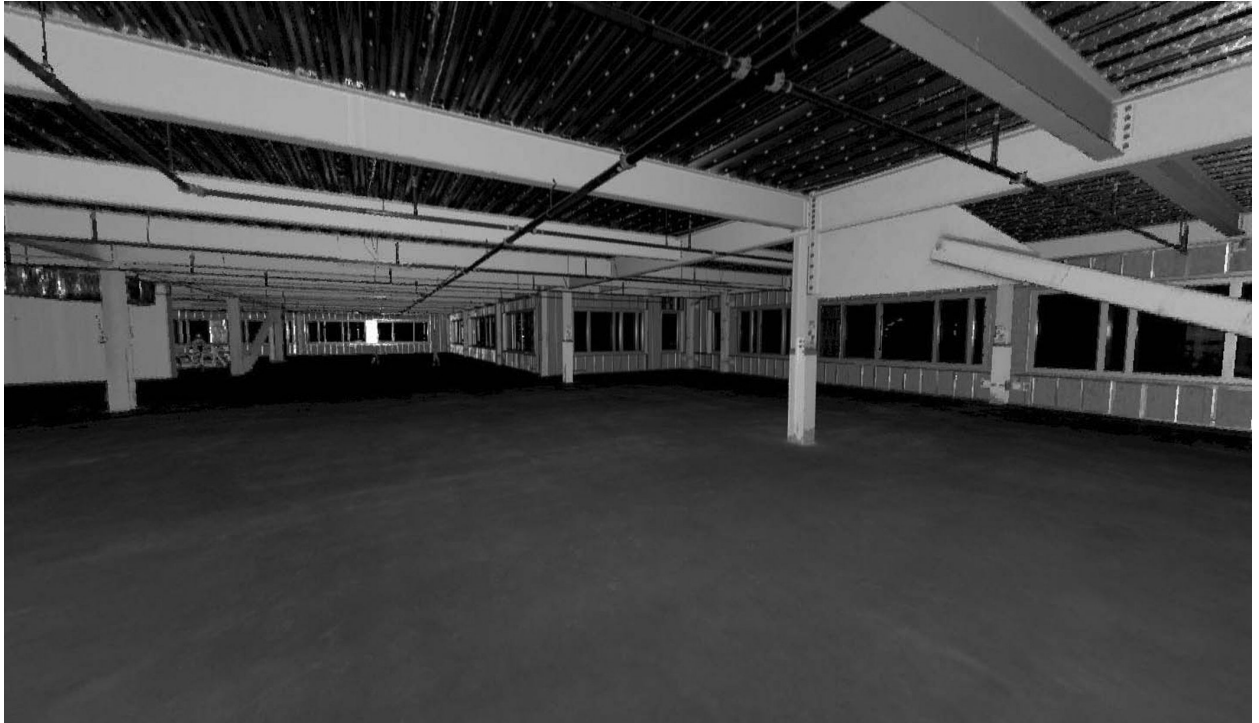
Figure 7.15 Trapelo existing conditions. Laser scan of building interior. Image courtesy of Tocci Building Companies and KlingStubbins
