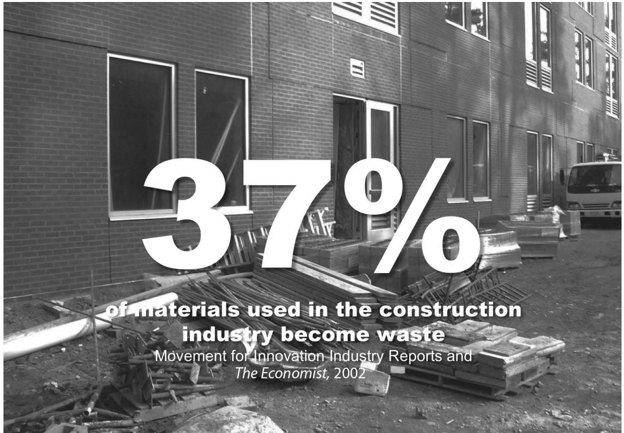
Figure 6.36 Thirty-seven percent of materials used in the construction industry become waste. Image courtesy of Tocci Building Companies and KlingStubbins
