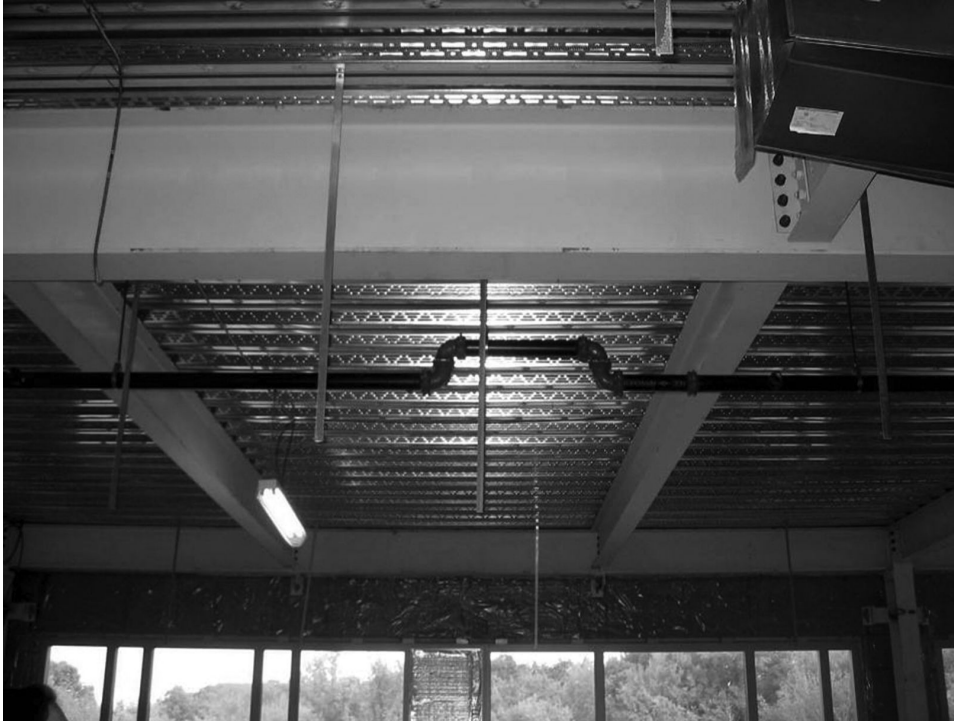
Figure 7.20 Photo of ceiling pipe condition. Image courtesy of Tocci Building Companies and KlingStubbins
