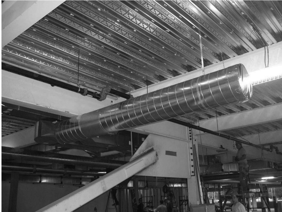
Figure 7.21 Photo of how modeled and coordinated ceiling pipe condition accommodates duct. Image courtesy of Tocci Building Companies and KlingStubbins
