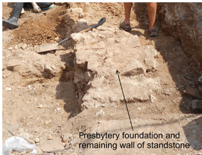
Figure 9.13 The exposed presbytery foundation and portions of the walls that are composed of sandstone and could be projected into the areas still preserved under the parking lot surface and tied to a GPR profile.
