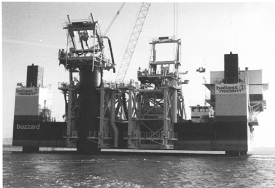
Fig. 9.24 Drilling equipment for sinking 3.50m OD precast concrete cylinder piles, Saudi Arabia-Bahrain Causeway
