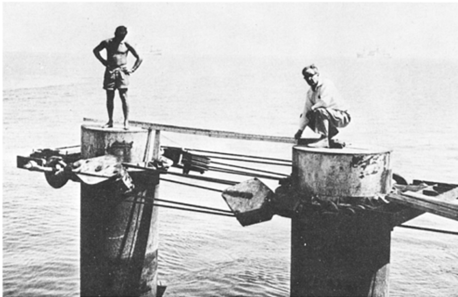
Fig. 11.18 Lateral loading test on two steel tubular piles forming part of breasting dolphin
