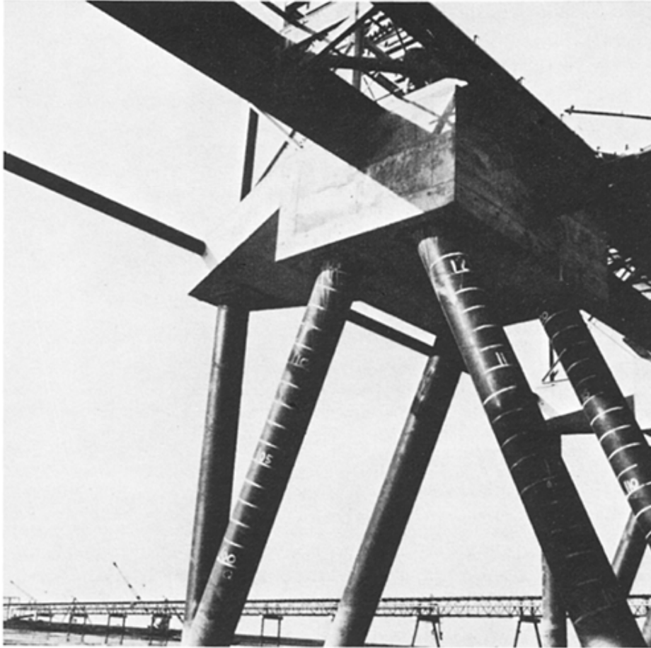
Fig. 8.2 Raking and vertical piles used to restrain berthing forces in bulk handling jetty
