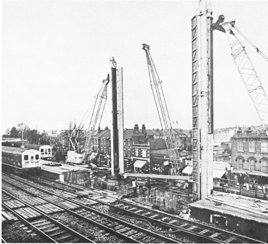
Fig. 3.20 Noise abatement tower used for 'Hush Piling' system
