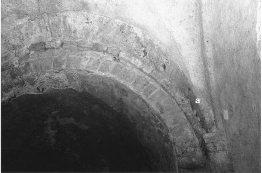
31. Aime, Saint-Martin, interior, southern transept, apse, arcade; (a) impressions left by lag boards above extrados of arch.
