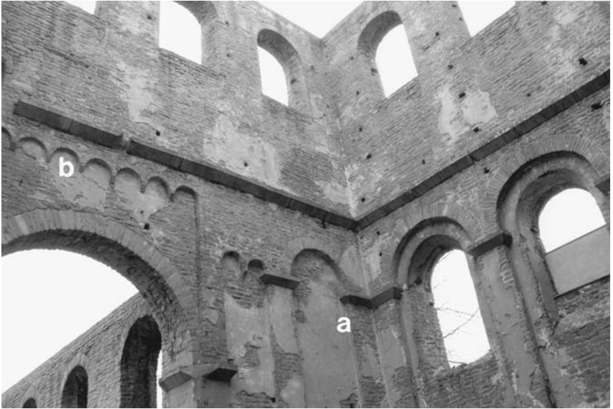
82. Limburg an der Haardt, abbey church, interior, north transept; (a) pilaster arcade; (b) corbel table.
