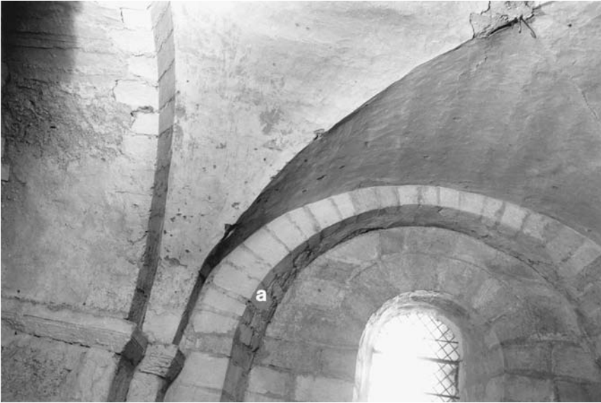
8. Auxerre, Saint-Étienne, interior, crypt, ambulatory, groin vault; (a) wide formeret stones at the base of the true vault.
