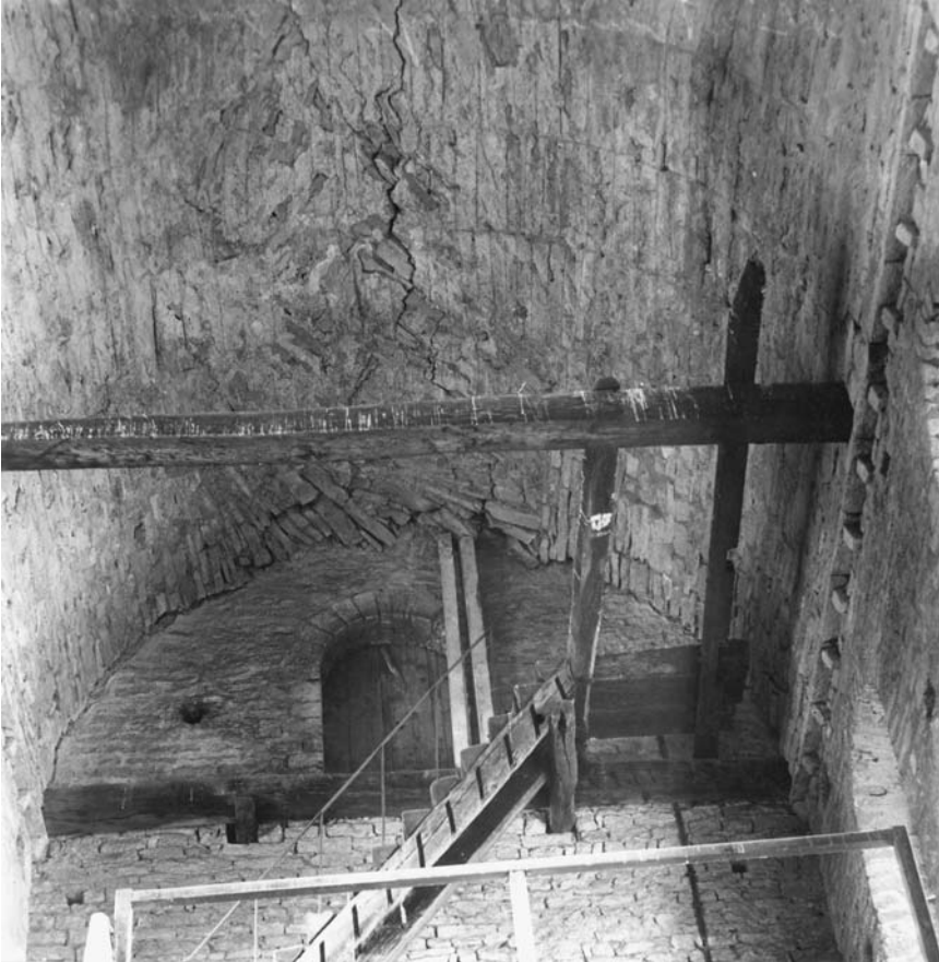
71. Tournus, Saint-Philibert, interior, upper narthex, central vessel, third bay, barrel vault, impressions left by lag boards in mortar (author's detail photograph from restoration file, Caisse Nationale des Monuments Historiques).
