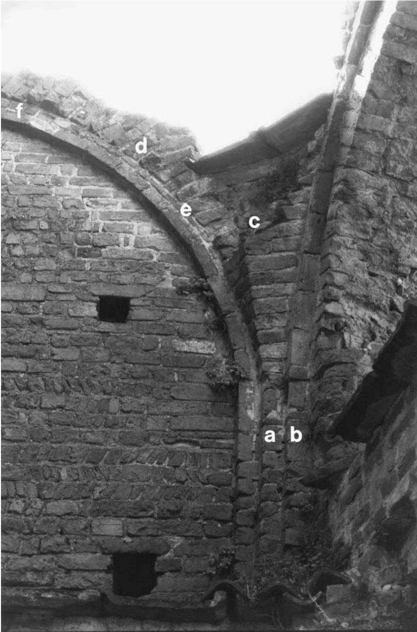
17. Lomello, Santa Maria Maggiore, nave, northern aisle, first bay, intersection of western and northern walls; (a) springing of the groin web; (b) springing of the formeret; (c) corbeled base of the vault; (d) radially laid bricks; (e) thin, horizontally laid bricks above formeret; (f) thick, horizontally laid bricks between formeret and crown of the web.
