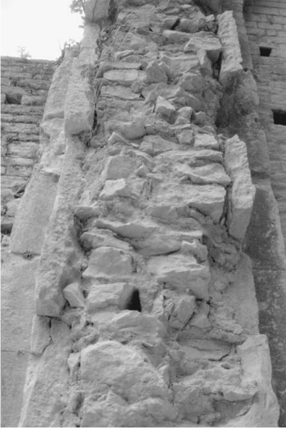
127. Cluny III, exterior, nave, southern aisle, bay six, buttress during reconstruction in 1996.
