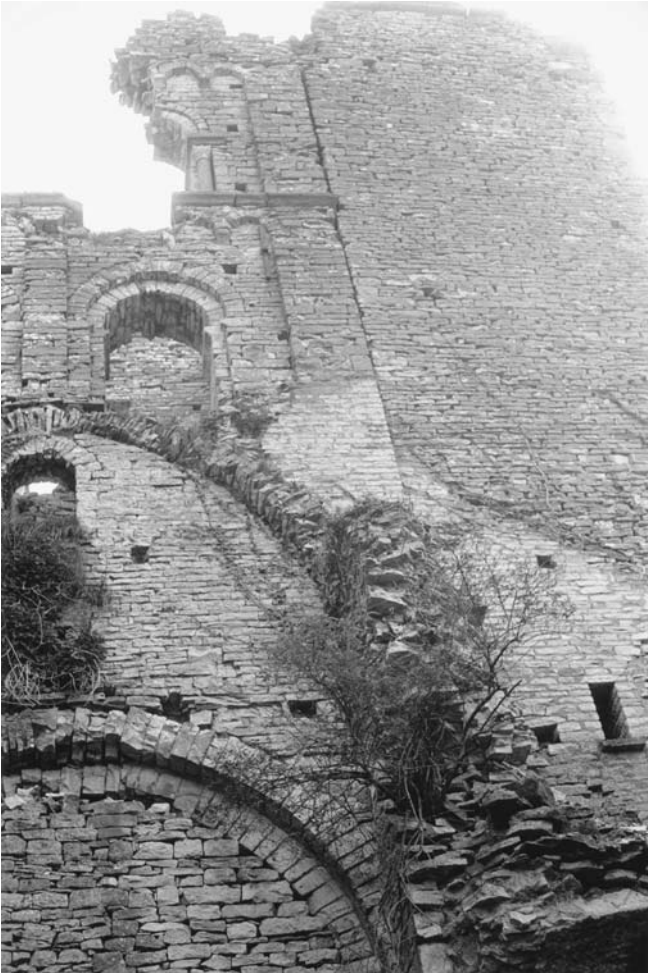
119. Saint-Hippolyte, priory church, interior, nave at cross- ing, detail of ruined central vault and elevation.
