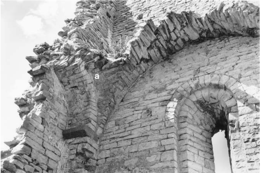
123. Saint-Hippolyte, priory church, interior, nave, northern aisle, western bay; (a) horizontally laid brick-shaped stones above extrados of transverse arch.
