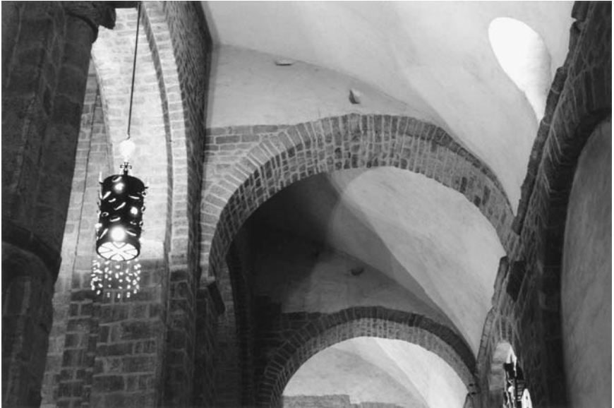
70. Elné, Sainte-Eulalie, interior, nave, northern side aisle, quarter-barrel vault, scaffold-beam holes in diaphragm arches.
