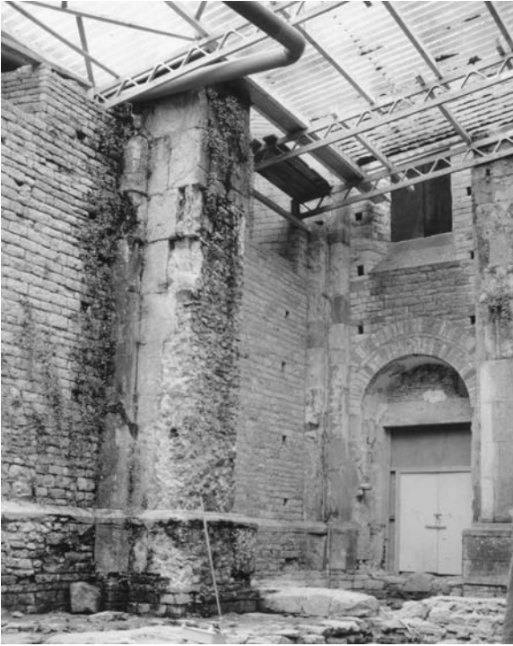
59. Cluny III, exterior, nave, southern aisle, bays six and seven, buttresses before reconstruction in 1996.
