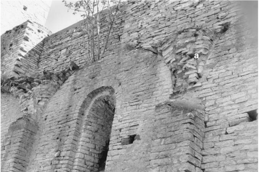
120. Saint-Hippolyte, priory church, interior, nave, southern aisle, ruined vaults; (a) brick-shaped stones in corbeled portion of vault course between groin webs.
