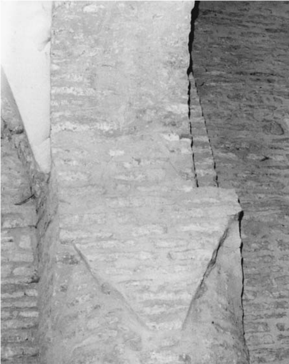
41. Chapaize, Saint-Martin, interior, nave, southern wall, westernmost arcade, intersection of aisle groin vault and impost with nave arcade, impost, and respond.
