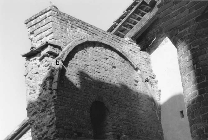
16. Lomello, Santa Maria Maggiore, nave, northern aisle, third bay, northern wall; (a) brick courses forming a semicircular platform for the formeret ; (b) formeret made of a double row of bricks.
