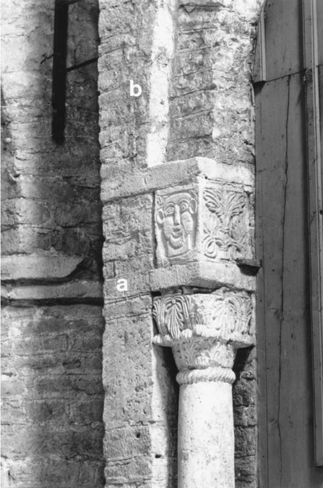
115. Tournus, Saint-Philibert, interior, upper narthex, eastern wall, central bay, portal, left jamb; (a) impost and jamb stone; (b) cover stones above portal voussoirs.
