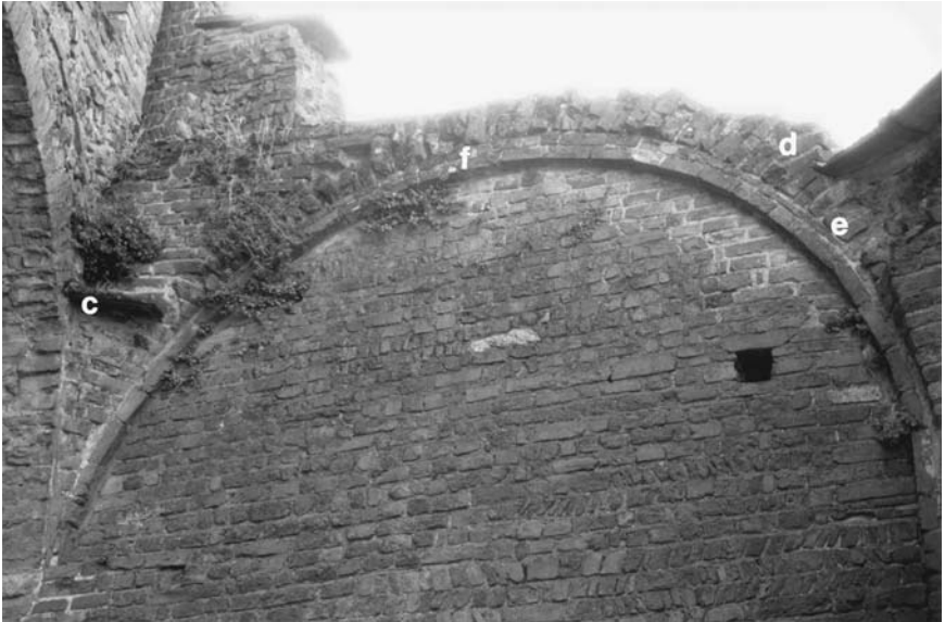
18. Lomello, Santa Maria Maggiore, nave, northern aisle, first bay, western wall; (c) corbeled base of the groin vault; (d) radially laid bricks; (e) thin, horizontally laid bricks above formeret ; (f) thick, horizontally laid bricks between formeret and crown of the web.
