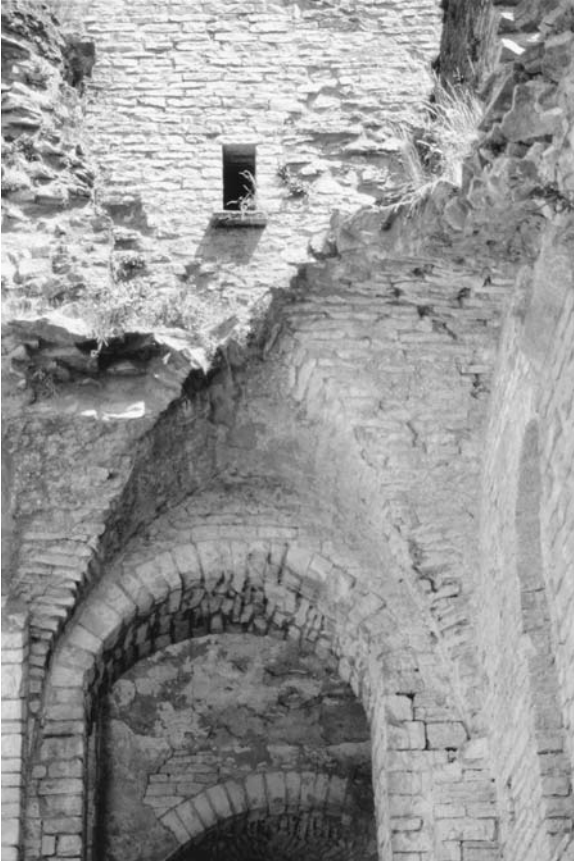
44. Saint-Hippolyte, abbey church, interior, nave, southern aisle, third bay, detail of ruined groin vault.
