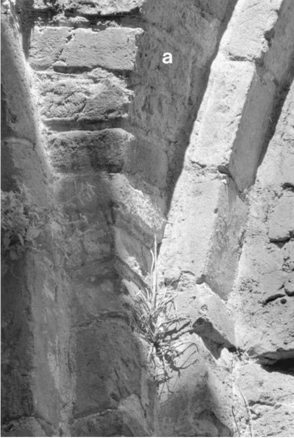
19. Lomello, Santa Maria Maggiore, nave, northern aisle, first bay, intersection of western and northern walls, corbeled base of the groin vault; (a) splayed brick running between two webs (detail of area shown in Fig. 17).
