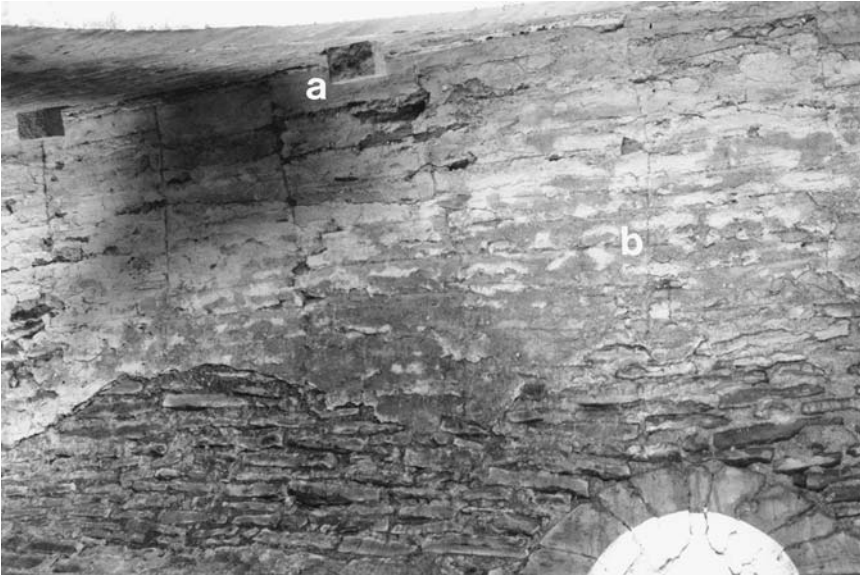
73. Brancion, Saint-Pierre, interior, nave, northern side aisle, half-barrel vault; (a) corbel block to support scaffolding; (b) impressions in mortar left by lag boards.
