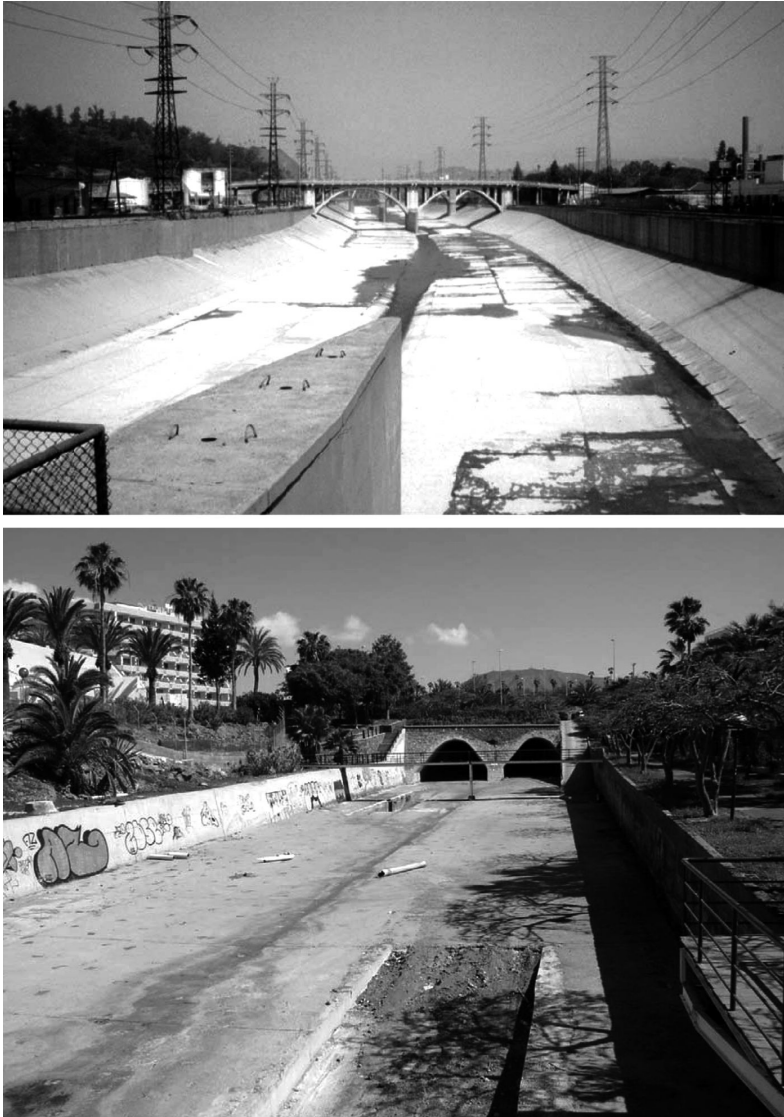
Figure 11.6 Channelization in the Los Angeles river (above) and Barranco del Rev Arena, south-west Tenerife (below)
