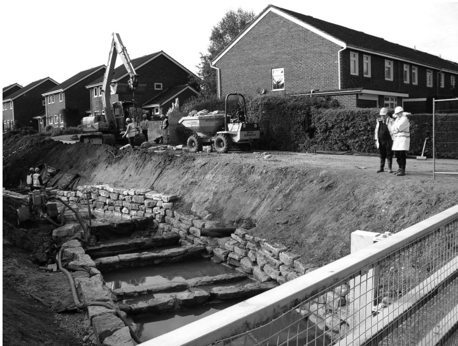
Figure 12.3 Tilmore Brook, Petersfield, UK – a restoration scheme devised to reduce flooding and erosion during construction (see Table 12.5; Brookes et al., 2005)
