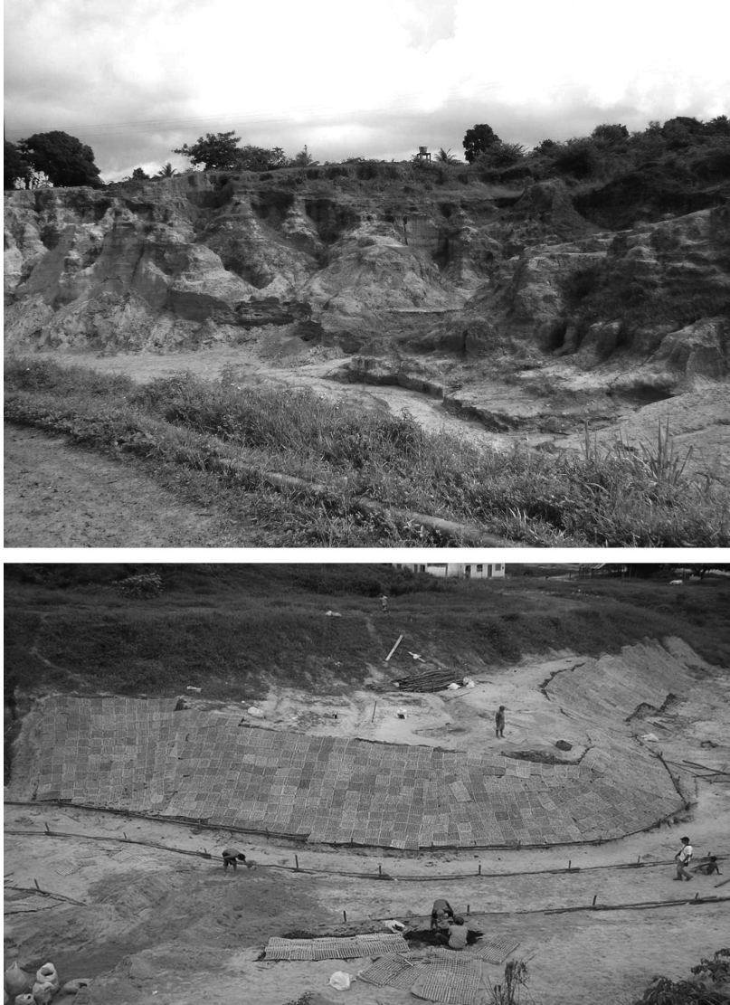
Figure 12.4 Sacavém, São Luís city, Brazil: (above) the gully system in 2006, where erosion has been monitored since 2000; (below) gully reclamation work in progress in São Luís, February 2008 with geotextile mats constructed from the leaves of local Buriti ( Mauritia flexuosa ) palms used for stabilizing gully head and slopes
