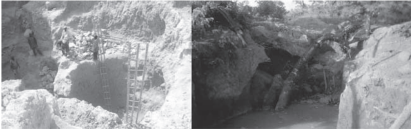
Photo 1. Artisanal gold mining well at Leggal Goro (depth ca. 80 m) and landslide bank (Takoutsi, 2009; Sinnota, 2004).
