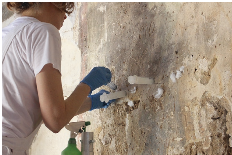
Fig. 12.5 During emergency stabilization. Injection of a pre-manufactured hydraulic grout in order to fill the gap between the detached plaster and the masonry and to re-establish adhesion
