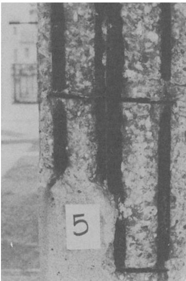
Fig.3. Bow-string r.c. bridge in Pavia(1935) corrosion of reinforcement.
