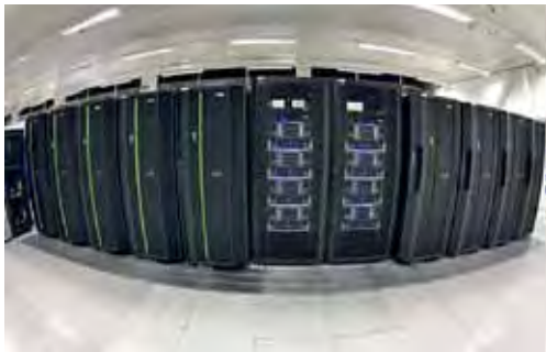
Figure 14.1 This IBM supercomputer is currently in use at the UK Met Office. Like ENIAC, modern supercomputers still fill a whole room, but can perform calculations at a much faster rate. (Photo: Met Office.)
