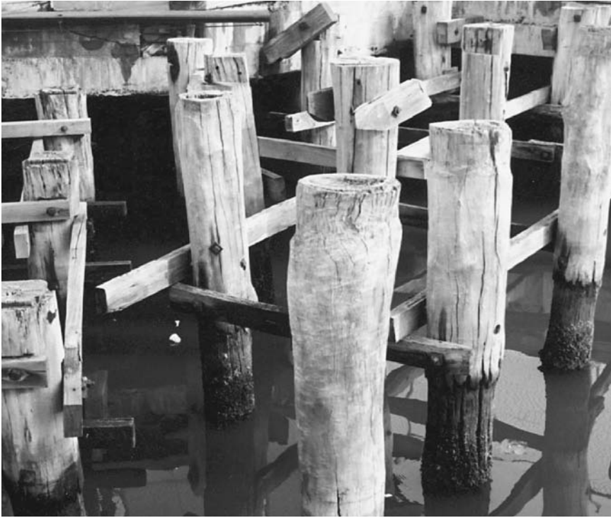
Figure 31. Paul Carter, Solution , “Forest in the Harbo*r, Timber Pilings, North Wharf” (Paul Carter, “ Solution: A public spaces strategy, Victoria Harbo*r, July 2002 ,” figure 24).
