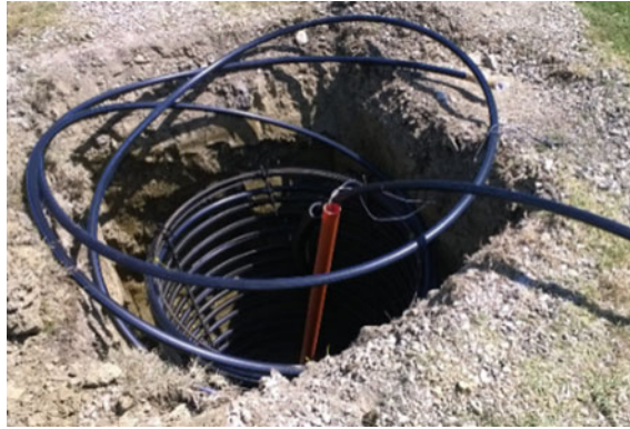
Fig. 2. The installation of the buried heat exchanger with the shape of a cylindrical basket whose performance is influenced by thermal properties of the soil
