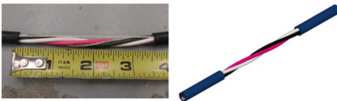
Fig. 7 (left) Damaged 3.5 in. section at the halfway point of a 100 ft. three-conductor shielded 600 V EPR cable; (right) corresponding ANSYS HFSS finite element model of damaged section
