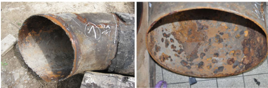
Fig. 1 Specimen cutting of an ND 500 \times 6.3 mm elbow for post service examination, after excavation and partial dismantling of the outside coating (left), and inner surface after cutting and before sand blasting (right)
