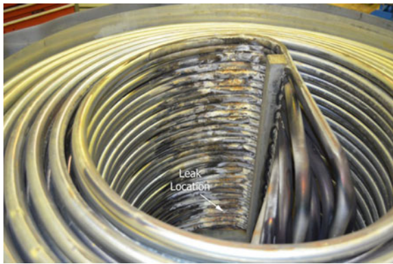
Fig. 4 The central cavity near the inlet side of the tube bundle. The tube #17 leak location is indicated
