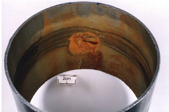
Fig. 1 Appearance of the inner surface of a leaking FFW pipe made from EN 1.4401 stainless steel. The reddish area is the lower side of the pipe in the piping
