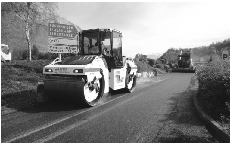
Figure 14.17 GB5 ® 0/14 mm with Budillon aggregate and SBS-modified binder Biprène ® 41 (proprietary composition) and 15% RAP near Chambéry. In-place density: 97%; modulus E^* (15 °C–10 Hz): 15,900 MPa.
