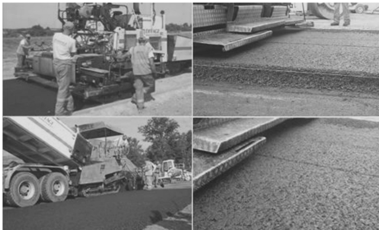
Figure 14.16 Paving GB5 ® 0/14 mm with Noubleau aggregates and 35/45 bitumen in the Tours area. In-place density: 96.4%; stiffness modulus measured in indirect tension configuration E^* (15 °C–10 Hz): 14,100 MPa.
