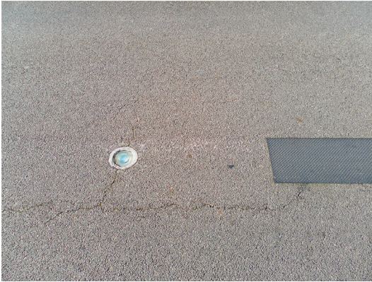
Figure 11.2 Example of cracked pavement made with vegetable binder.
