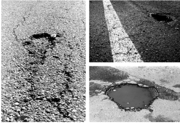
Figure 10.1 Deteriorated pavements due to water-induced damage. (a) Raveling caused by segregation. (b and c) pothole formation.
