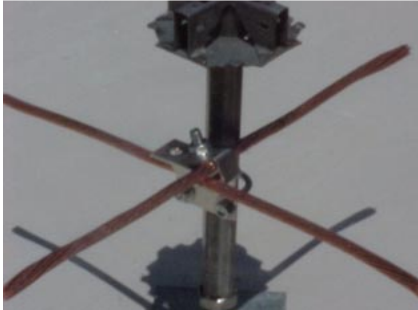
Figure 4-50—Typical cellular raised floor's pedestal post and later-made ground connections to/from it
