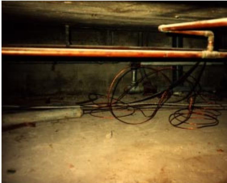
Figure 10-4—Excessive grounding conductor coil
