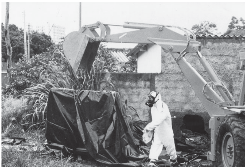
FIGURE 12.3 Demolition of a contaminated home. Due to the extensive contamination by radioactive cesium-137, this home had to be demolished. The entire contents and the layer of topsoil were taken to a landfill designed to accept radioactive materials. (International Atomic Energy Agency)
