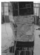
Figure 14. Failure pattern of column SP-3 (after stripping of bands).
