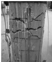
Figure 4. Failure pattern of column DP-2 (after stripping of bands).
