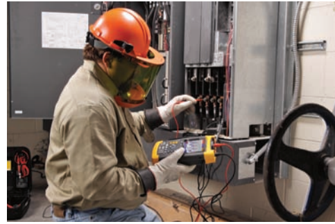
Figure 10-30 Taking measurements on a VFD.
