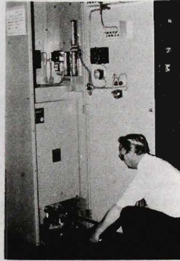
(b) Breaker being withdrawn from its cell
