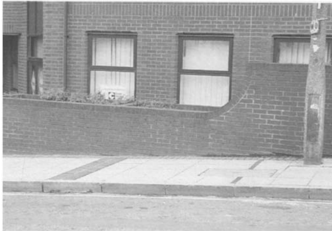
Figure 4.1 General view of brick parapet wall, coping and walling in the same porous brick. This shows algae staining concentrated on the coping but extending down the wall face.
