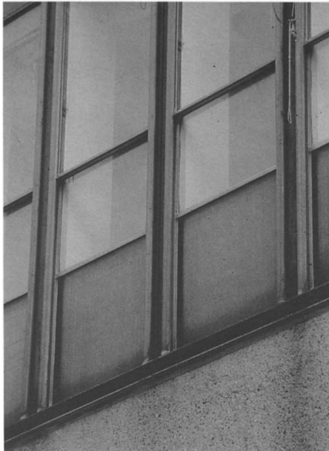
Figure 4.42 Detail at junction of curtain walling and concrete plinth showing concentrated staining at mullion positions.
