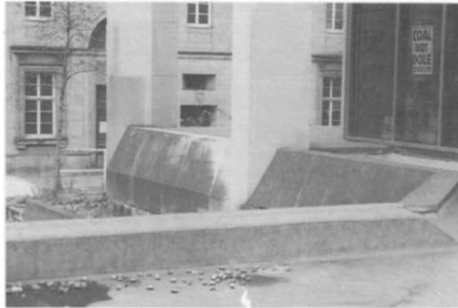
Figure 3.3 Detail showing extensive algae growth to the surface of the cladding around the base of the building. Here water flow from the top of the parapets and hardstanding has been directed over the face of the panels. The elevation faces north.
