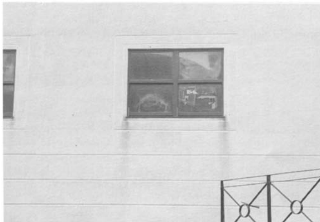
Figure 4.36 Detail of Figure 4.35. This staining has probably been enhanced by the breakdown of the sealant around the frame depositing substances on the walling.
