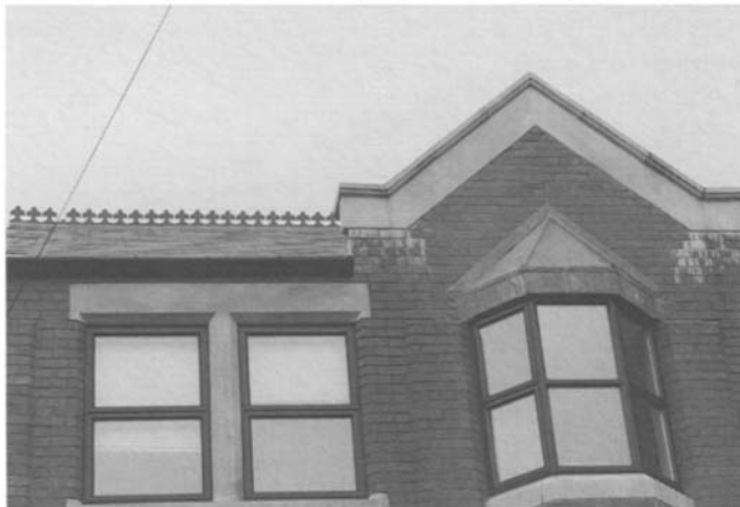
Figure 4.17 Staining caused by inclined copings. This two-year-old feature shows both the disfigurement of lime and premature staining.
