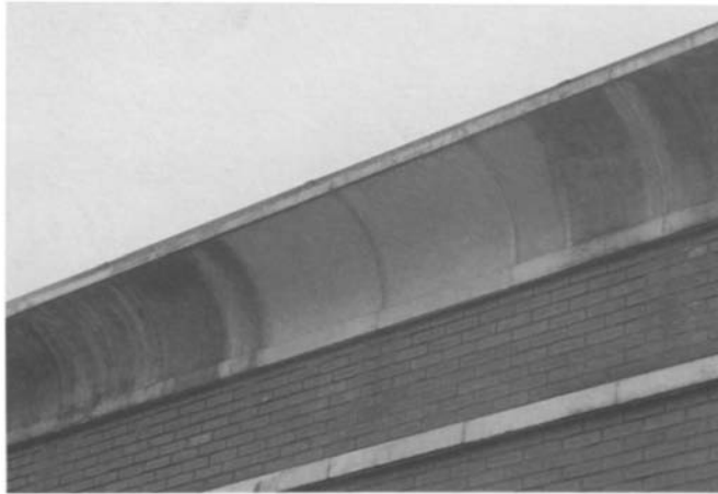
Figure 4.56 Detail of Figure 4.55 showing the clean surface of the two cornice units with throatings compared to those without.
