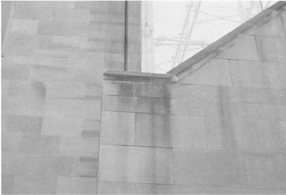
Figure 5.6 The inclined cills beneath the glass cladding concentrated the water flow at the change in inclination.
