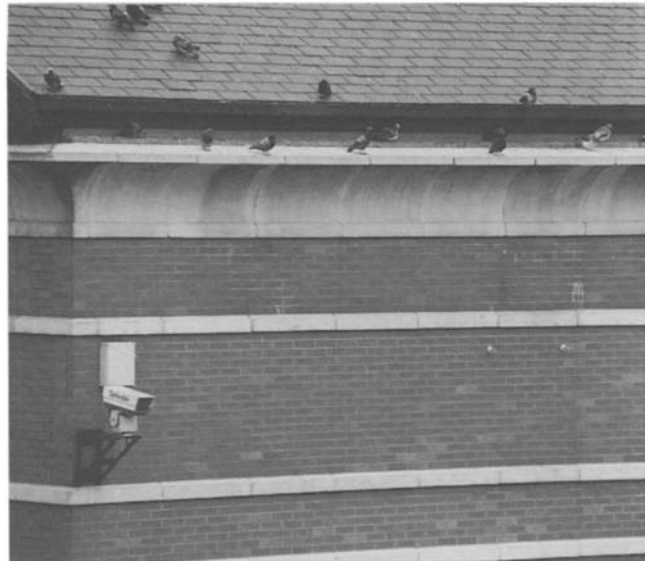
Figure 4.54 General view of the cornice and string courses showing the beginnings of staining concentration following the joints.
