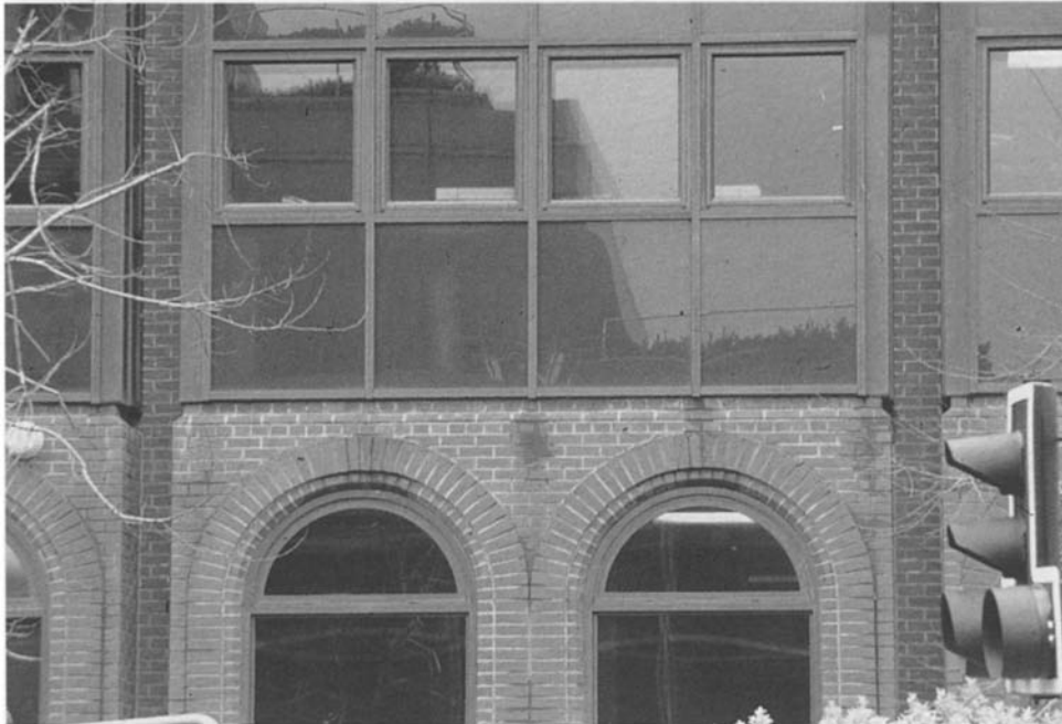
Figure 4.43 Staining at mullion positions where cladding is less pronounced.
