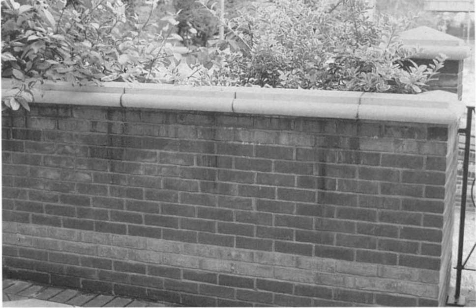
Figure 4.67 The coping units have rounded edges with no throating beneath allowing water to flow down the surface of the walling below.
