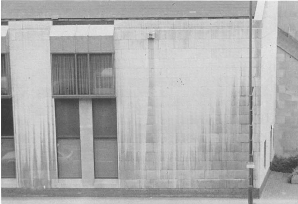
Figure 5.8 Detail of Figure 5.7 showing the sheltering effects of a protruding detail on the wall surface.
