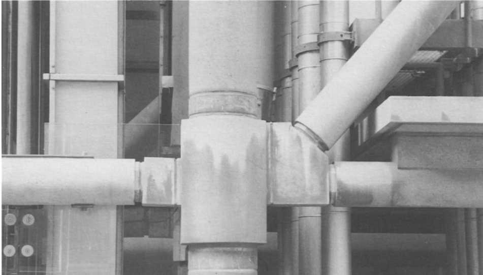
Figure 5.3 Detail of a junction to the exposed concrete frame of the Lloyds building showing uneven washing and staining.
