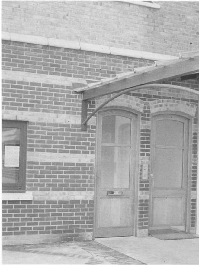
Figure 4.72 The canopies above the main entrances have no guttering which allows rain splashback to stain the walls at low level.
