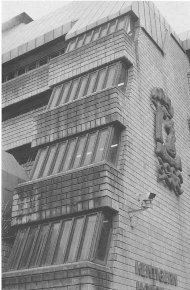
Figure 3.5 Detail of Figure 3.4 . Water was allowed to flow off the metal roof and onto each glazed area cumulating as it travelled downwards. There was no gutter or drain to minimize the flow which resulted in extensive algae growth increasing in intensity at lower levels.
