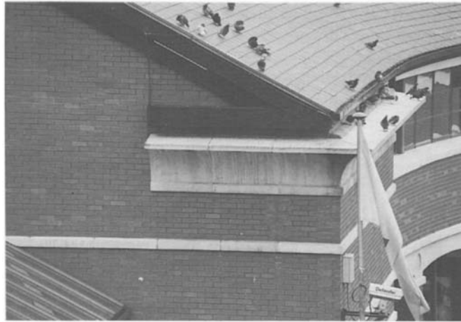
Figure 4.53 Detail of strong visual cornice units. Note that the side facing the camera has been netted to prevent pigeon roosting while the other has not.
