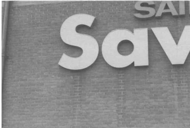
Figure 4.49 Detail of Figure 4.48 showing staining below lettering that is fixed flush to the wall.
