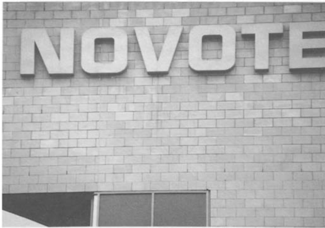
Figure 4.47 Detail of lettering fixed flush to the wall surface. Evidence of early staining especially below the 'V'.
