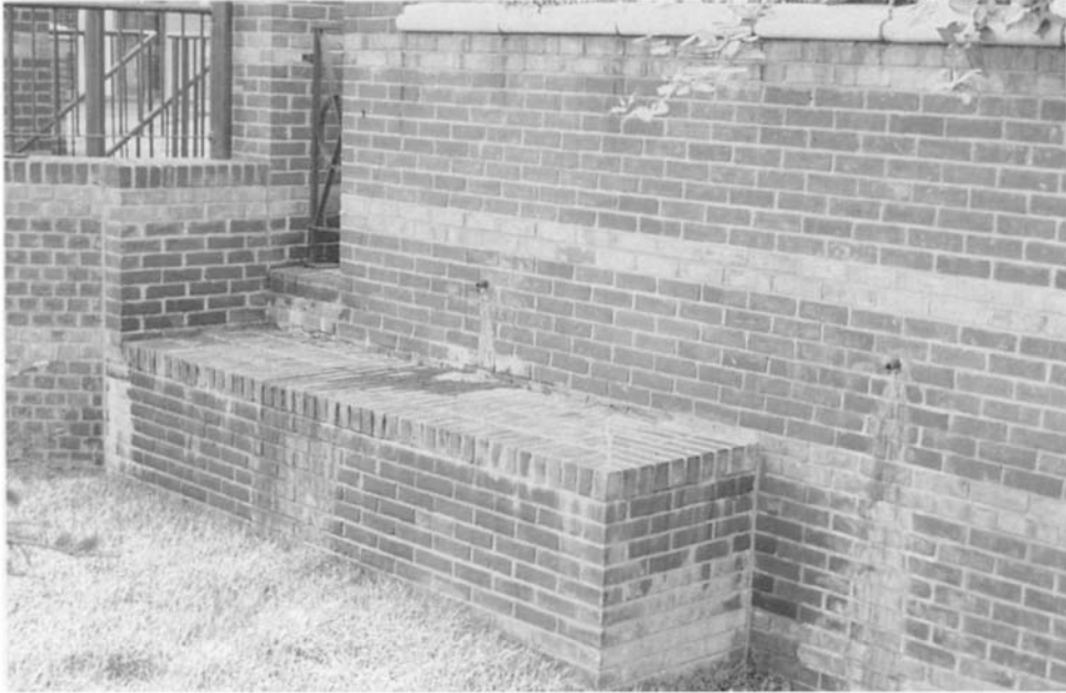
Figure 4.70 An isolated brick plinth has been badly stained by water flow from the hardstanding above and spitter pipes draining the adjacent planters.
