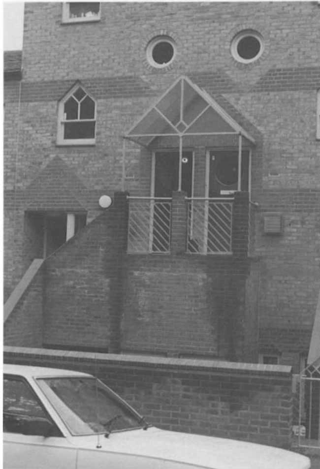
Figure 4.85 This glass-covered canopy has no guttering system and discharges over the flat entrance area below. Because there is no raised upstand on this balcony the water flows over the walling below causing staining.
