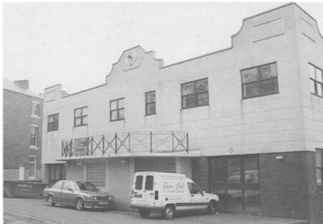
Figure 4.35 Recently refurbished building showing 'moustache' staining.
