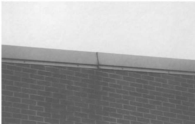
Figure 4.32 Detail of Figure 4.31 showing high levels of water flow at junction of adjacent units.
