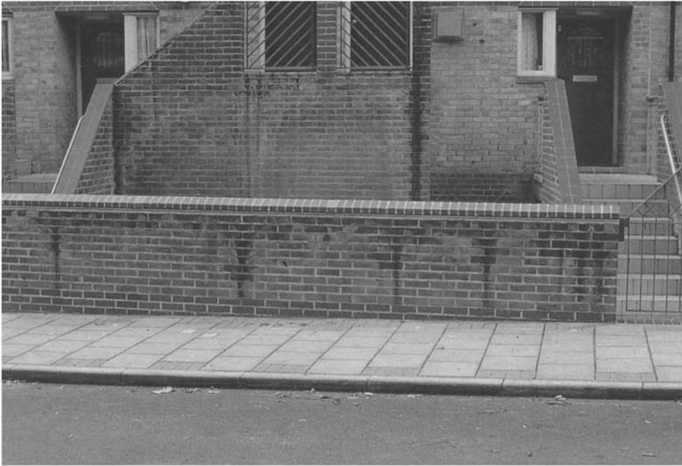
Figure 0.2 The boundary wall was particularly badly affected.
