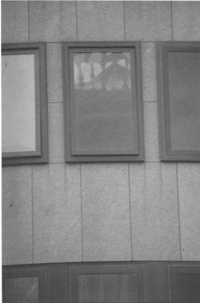
Figure 4.44 Staining caused by sealant or gasket migration.
