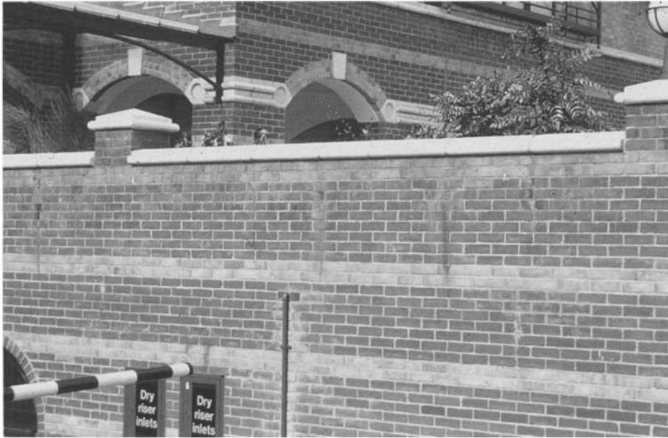
Figure 4.68 Conspicuous joint staining has affected all parapet walls.
