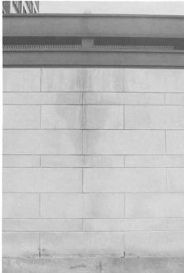
Figure 3.8 Detail of roof/cladding junction. Run-off from the roof components was allowed to flow over the stone depositing green/grey stains on the face.
