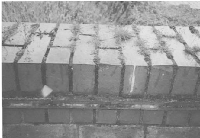
Figure 4.2 Brick coping with relatively impervious bricks and porous mortar. Algae and moss growth is quickly followed by grass and other higher-order plants. Tile creasing is also shown that has been laid flat without weathered mortar pointing allowing moss and lichens to become established.
