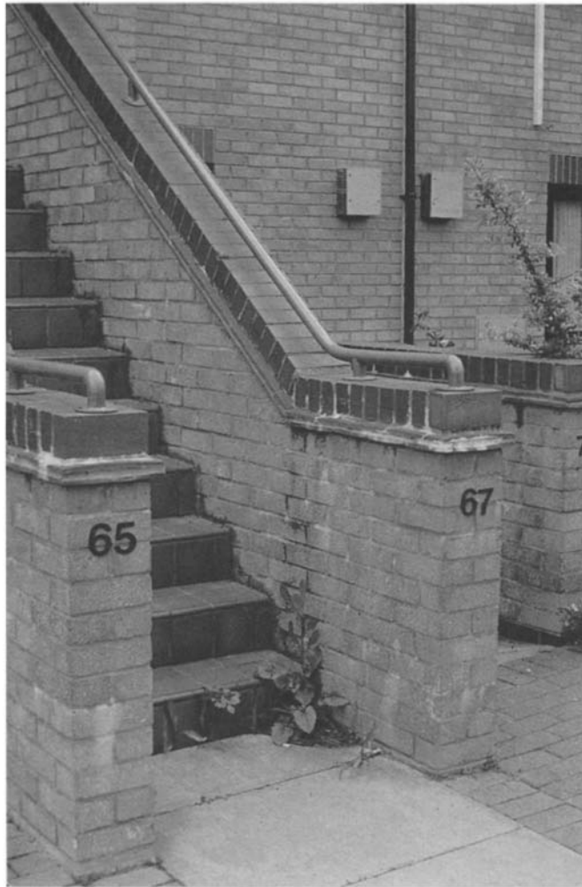
Figure 4.82 Brick on edge coping and tile creasing fails to prevent the increased flow of water at the change in inclination. Lime staining is also evident here.
