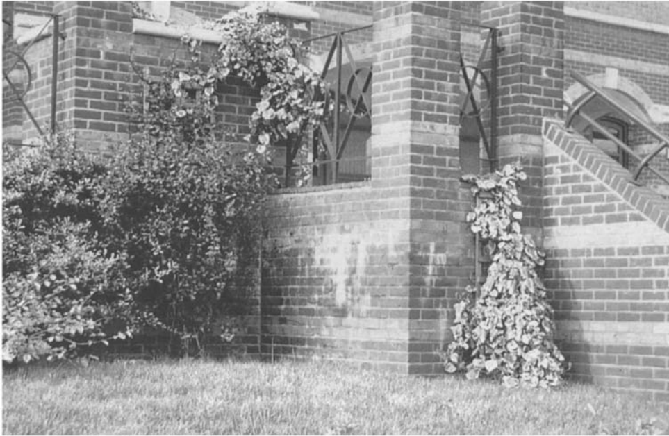
Figure 4.69 In many areas poor damp proofing behind retaining walls has allowed intense lime staining to disfigure the brickwork.
