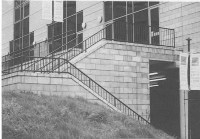
Figure 4.84 The broad flat coping at high level allows water to flow down the face of the prominent elevation disfiguring the reconstituted stone blocks.
