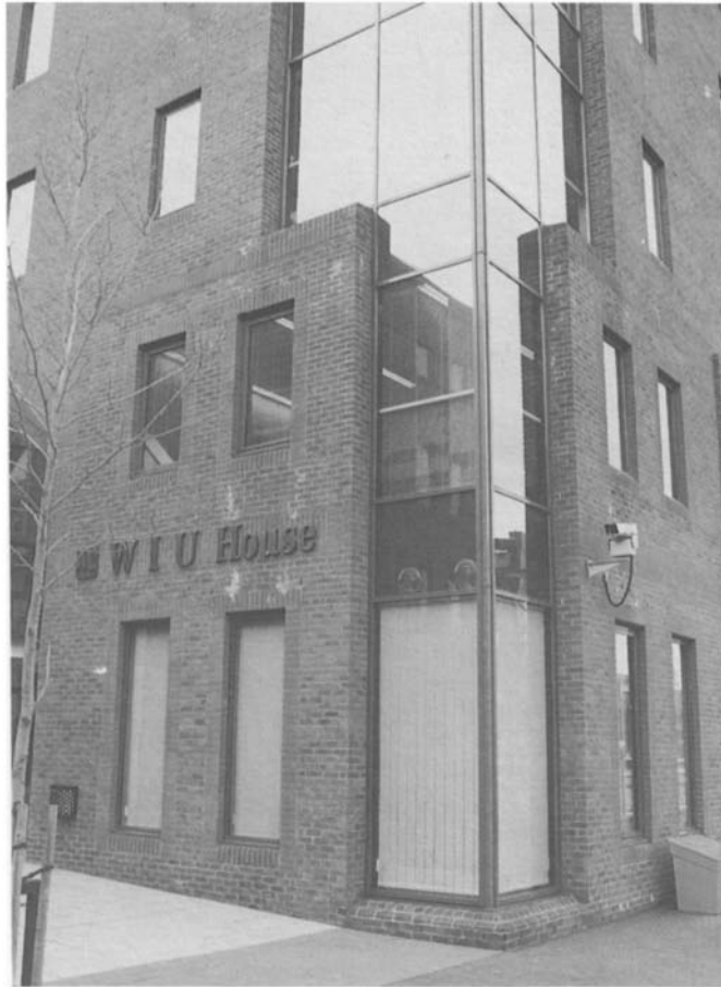
Figure 4.38 Detail of the bottom two storeys showing the lack of any cills at the glass/brick cladding junction.
