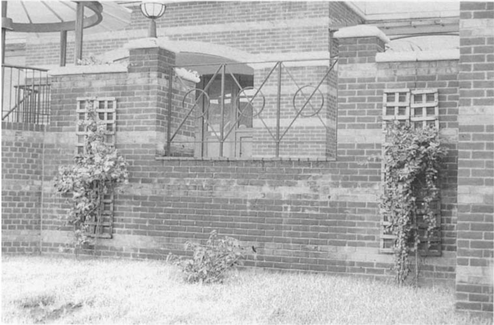
Figure 4.64 Much of the hardstanding is drained by discharging over the face of the retaining walls.
