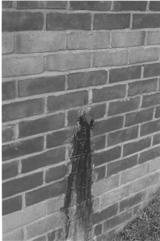
Figure 4.71 The watertightness of virtually all spitter pipes was defective allowing ugly water flow down the face of the brickwork. Here the water is draining around the pipe rather than through it.
