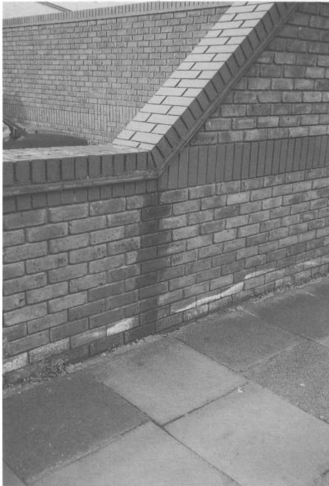
Figure 4.7 The inclined boundary wall with a non-porous coping directs coping run-off directly on to the tile creasing. This flows down the slope and because of the lack of an effective throating beneath the creasing there is a concentrated water flow and consequent staining at the change in direction.
