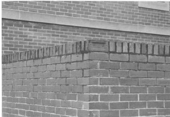
Figure 4.4 Detail of Figure 4.3 showing the concentration of staining to mortar joints through algae and moss growth. Because the mortar is more porous than the bricks, its surface remains damp and provides a good growing medium.
