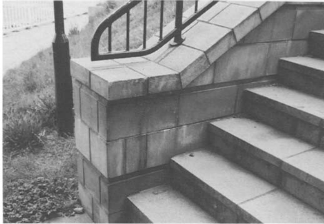
Figure 4.81 The broad flat surface of the parapet wall to this staircase (see Figure 4.80) allows large amounts of water to flow down to the base of the stair and discharge over the walling.
