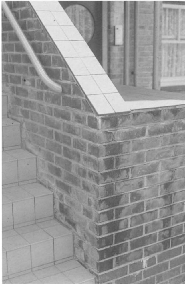
Figure 4.83 The 'clean lines' of this design has resulted in the absence of any form of overhang/throating allowing water flow to affect the face of a brick-built bin store below.
