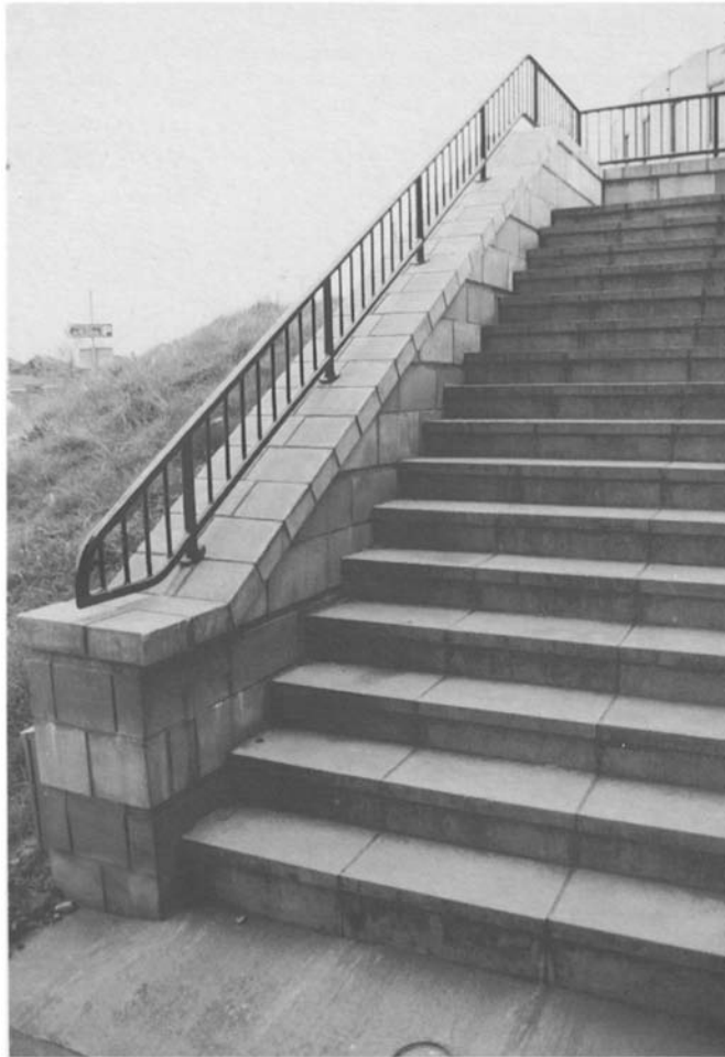
Figure 4.80 Staircase where the handrail and balusters have been fixed through the coping construction. The junctions of the main posts and the copings are very difficult to waterproof, potentially allowing water to stain the walling below.
