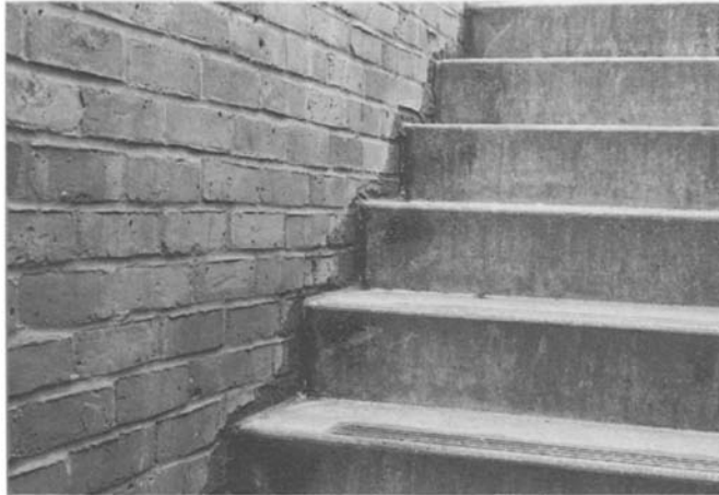
Figure 4.79 Longer exposure to the elements will lead to algae and moss growth at the junction of the steps and brick wall.
