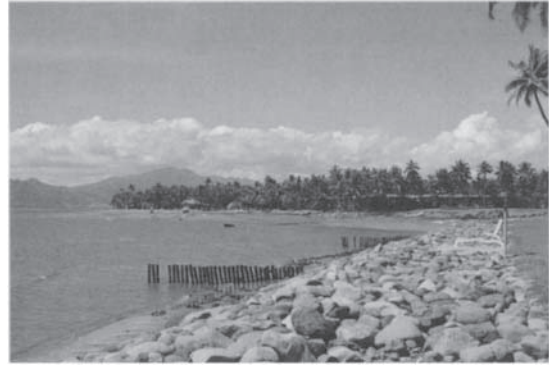
Plate 4.5: Coastal erosion measures on Denarau Island, Fiji, to prevent the unstable former mangrove swamp from being denuded
