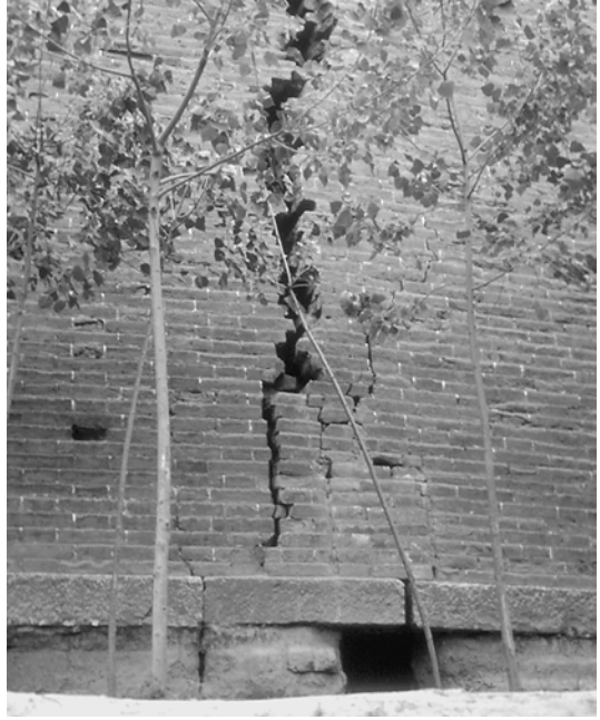
9-5. Damage to a compound wall, resulting from a severe earthquake in the 1970s in Sian, China (photo by the author, 1977).
