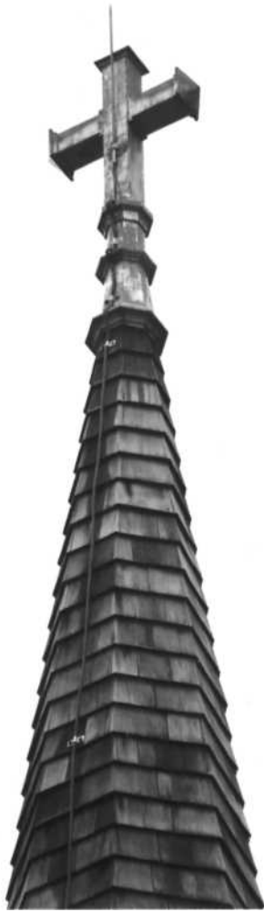
Figure 3. A cross with lightning rod attached. Location: Town of Oak Bluffs on Martha's Vineyard, Massachusetts (photograph courtesy of William Waterway).
