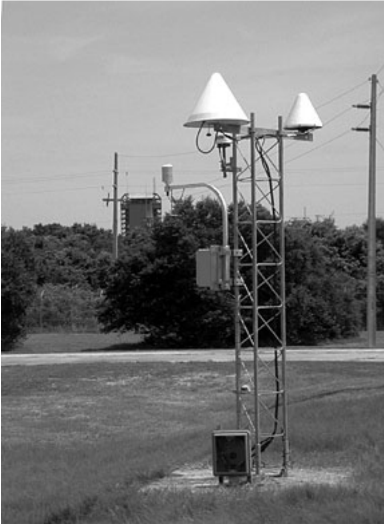
Figure 8. GPS-IPW installation at the U.S. Coast Guard Differential GPS site at Cape Canaveral Air Force Station.
