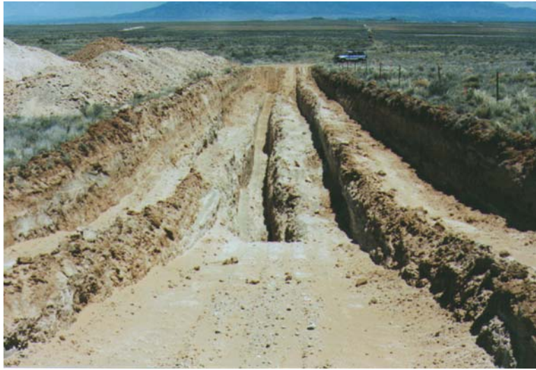
Figure 2A.27: Photograph of a trench dug by wheeled loaders, with a central slot dug by a trackhoe. The slot had previously been shored with hydraulic shoring, but those were removed by the time this photo was taken, just prior to backfilling. West Trench, Calabacillas fault, Albuquerque, New Mexico (McCalpin and Harrison, 2000). Photograph taken by J. P. McCalpin on June 1, 1999.
