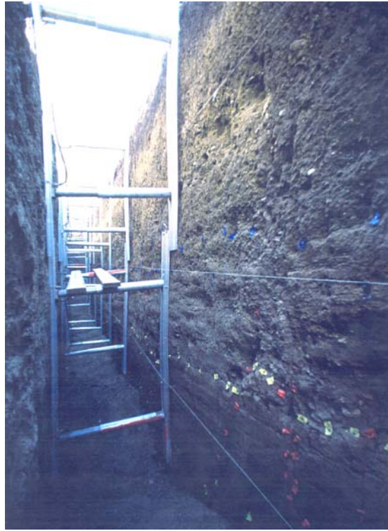
Figure 2A.23: Photograph of the interior of a 0.9 m-wide, 4.3 m-deep single slot trench (Kaysville trench, Wasatch fault zone, Utah; see McCalpin et al. , 1994). Hydraulic aluminum shoring supports, each 2.15 m high, are stacked in two tiers. Sediments exposed in walls are fine-grained graben-fill sediments; red markers show faults, yellow and blue markers show stratigraphic units.
