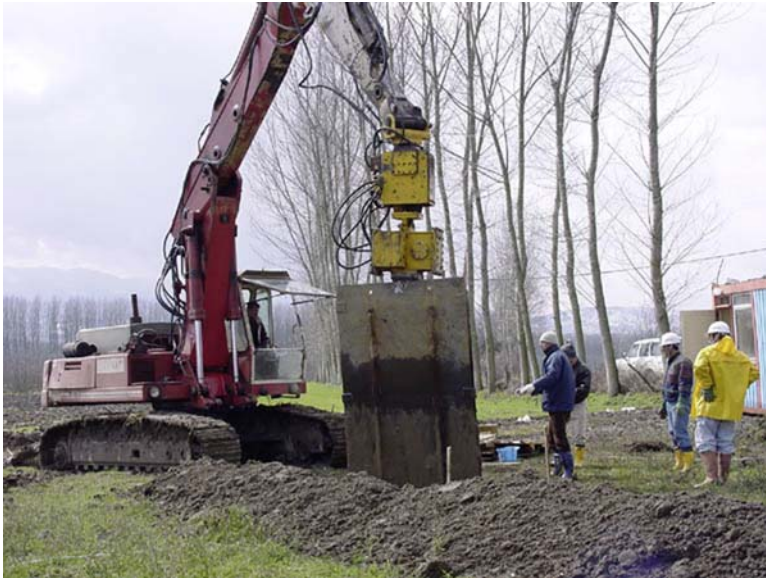
Figure 2A.47: Photograph of a wide geoslicer mounted on a trackhoe arm with a hammering attachment. Photo courtesy of K. Okumura.
