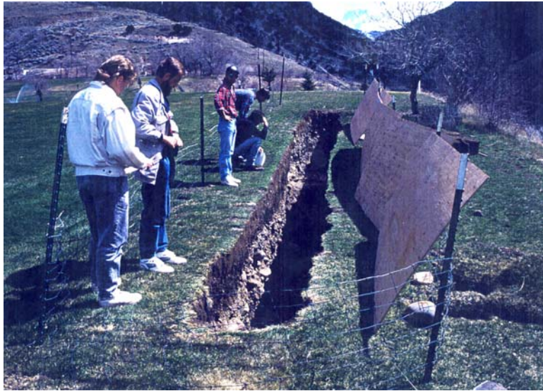
Figure 2A.24: An example of “clean trenching” in a developed area (golf course). The turf at this site was cut out and rolled (lower right) and all material excavated by a small backhoe loader was placed directly in a dump truck and hauled off-site. The trench was then fenced and covered with plywood sheets (at right) when loggers were not present. The trench was logged simultaneously with golf course use, and neither activity interfered with the other. However, golfers who hit balls into the trench were assessed a two-stroke penalty.
