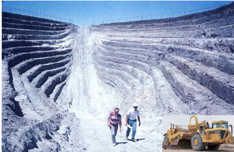
Figure 2A.28: Multibench trench excavated by scrapers. The trench sidewalls are composed of 13 vertical walls each 1.5 m high, separated by 12 horizontal benches 1.5 m wide; total depth is ca. 20 m, total volume ca. 23,000 m 3 . Total excavation cost was about US $100,000 (1995 dollars). The trench was excavated to determine the origin of a 20-cm-wide ground fissure in an area of proposed commercial development at Lakeview Hot Springs, southwestern Riverside County, California. The fissure proved to be the surface expression of an old hot springs vent and was unrelated to previously suspected faults or to local differential settlement. From McCalpin and Shlemon (1996).
