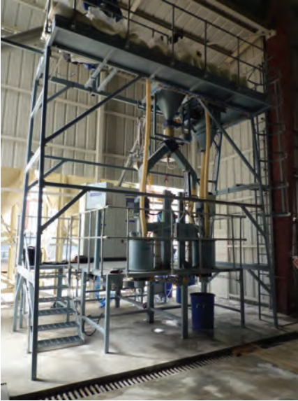
Figure 4.2 Integrated automated batching/mixing plant. (Courtesy of L. White.)
