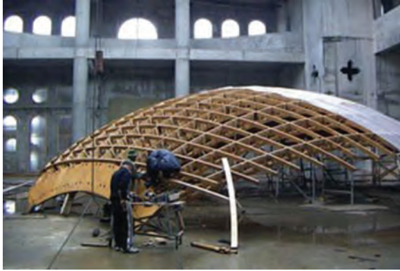
Figure 4.10 Mould for production of a prototype GRC panel forming a section of a large dome. (Courtesy of the iGRCA.)
