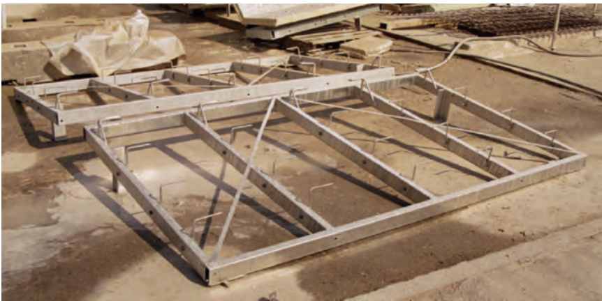
Figure 7.4 Thin-walled hollow sections in galvanised steel with anchors, ready for the assembly of a stud-frame GRC panel.
