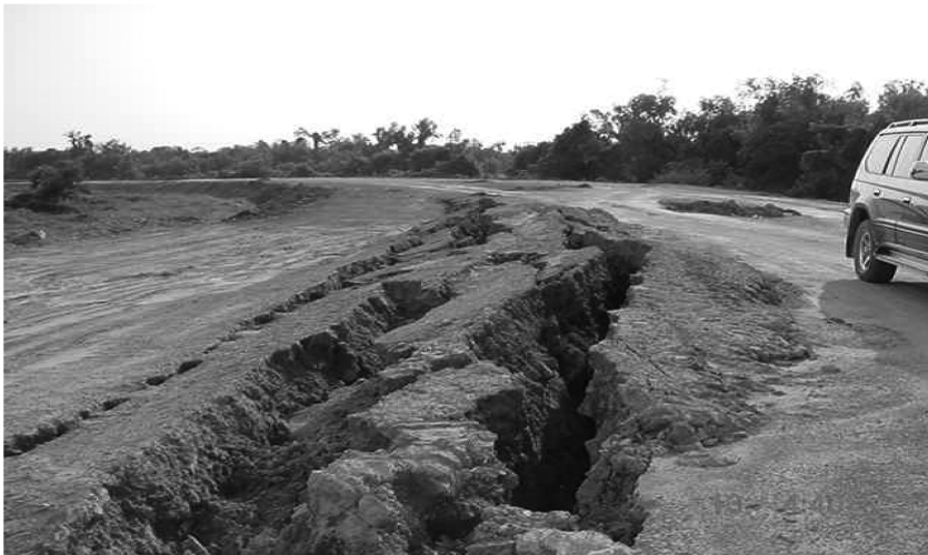
Figure 6.1 (a) Bearing capacity failure in peat; (b) embankment crack (after Hussein and Mustapha, 2003).
