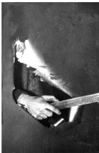
Figure 5.28. Wear damage of drying line components after five months of service – through hole in a large-size rectangular section air conduit
