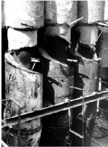
Figure 5.27. Cyclone battery being repaired; in the middle part of the middle cyclone there is a coated patch welded in place of the cutout
