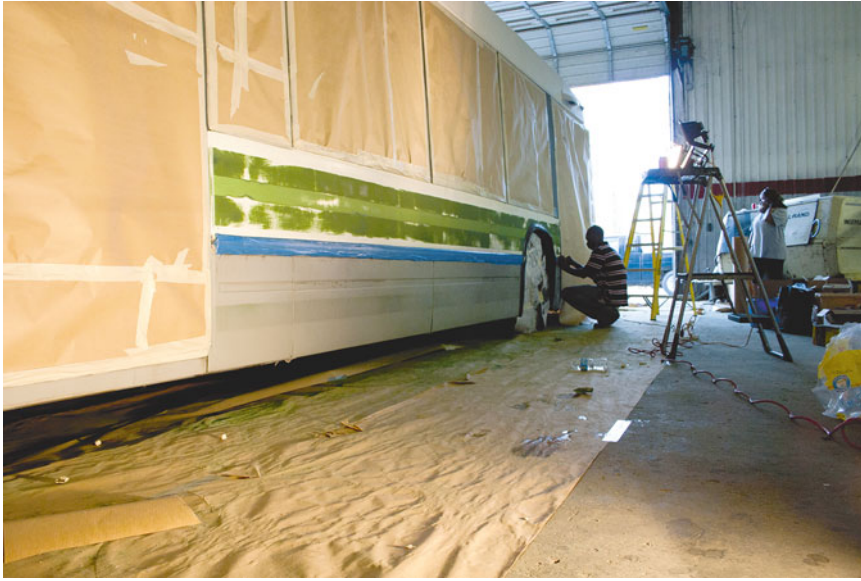
Fig. 30.2 Initial phase of the bus transformation in the General Plumbing Company’s Main Warehouse
