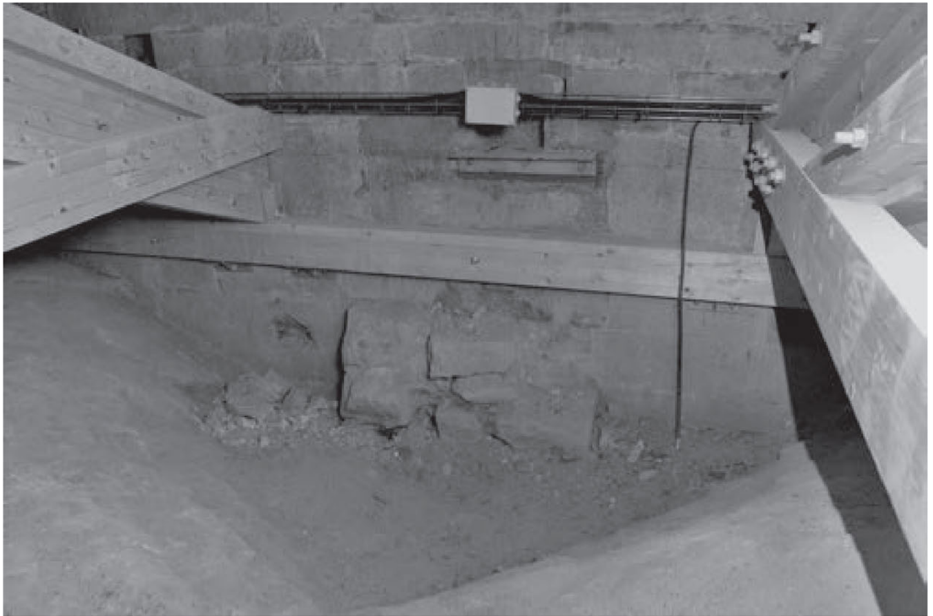
Fig. 9. Jaca Cathedral, springer of an arch over the modern vault of the north aisle (photo author)
