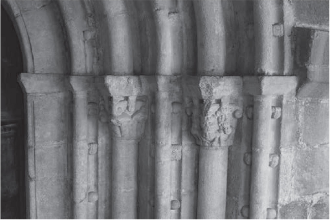
Fig. 5. Entrance to the church: detail of the little heads on the archivolts (photo authors)
