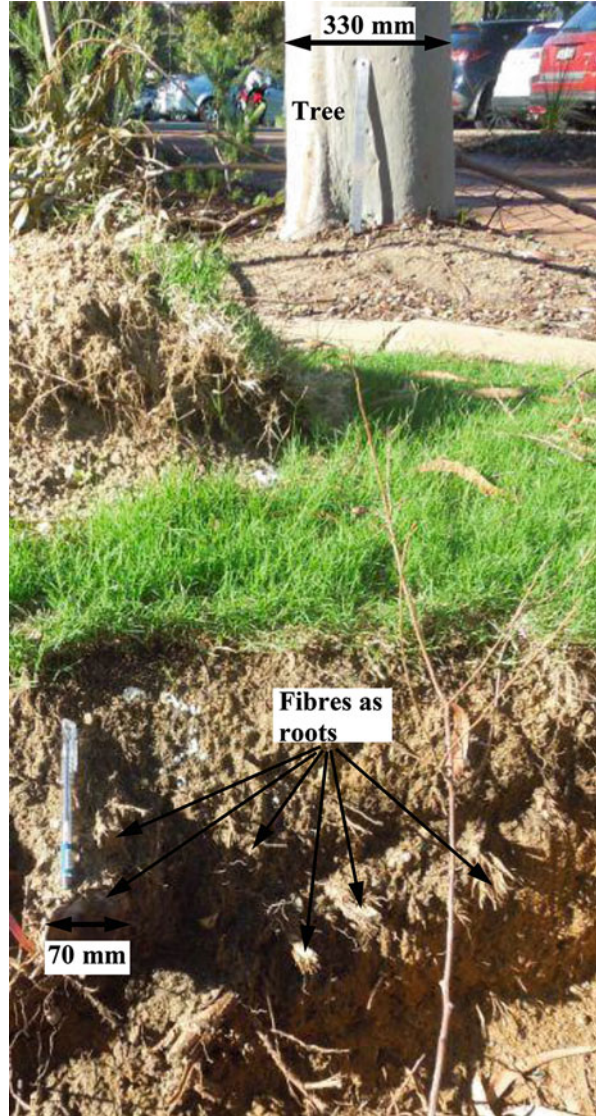
Fig. 2.1 Foundation soil reinforced randomly with natural root fibres (visible in an excavated trench closer to the tree) supporting a tree
