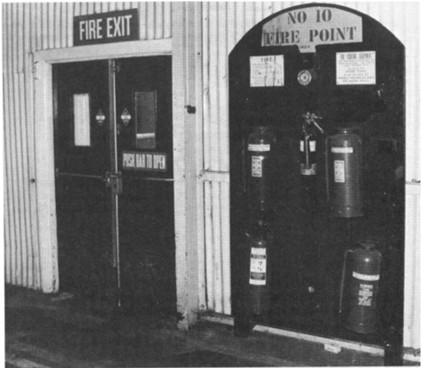
Figure 2.16 Clear unobstructed fire point. (Courtesy Reed Medway Sacks Ltd)
