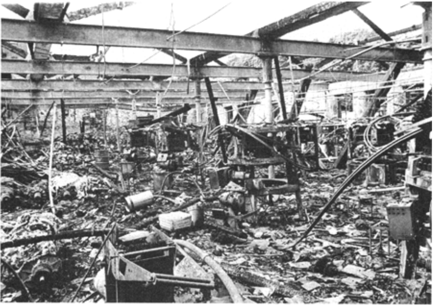
Figure 2.5 Aftermath of fire in textile mill. (Courtesy Huddersfield Examiner)
