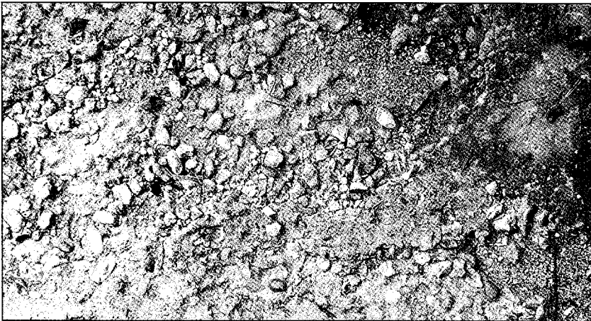
Figure 4.7: Freeze-thaw scaling due to de-icing salt exposure.
