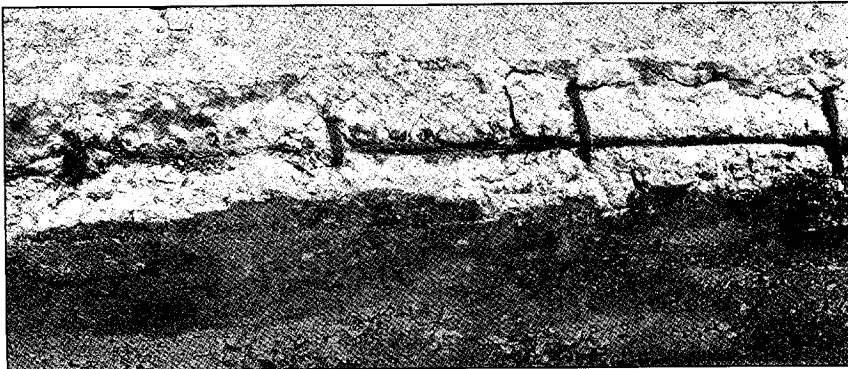
Figure 3.3: Spalling due to chloride-induced corrosion. Marine exposure.
