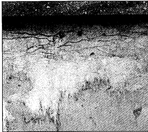
Figure 4.5: Deterioration due to freeze-thaw attack at the top of a concrete wall.
