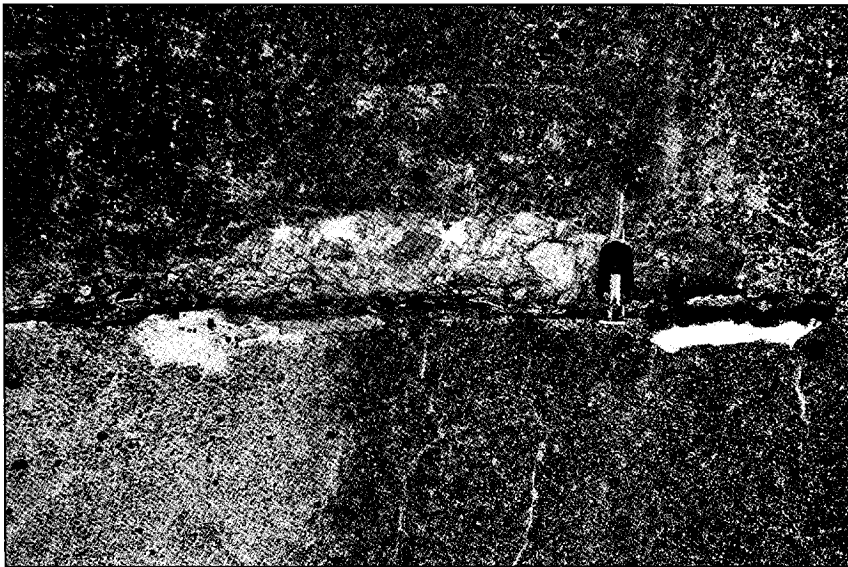
Figure 4.3: Spalling caused by freeze-thaw attack.
