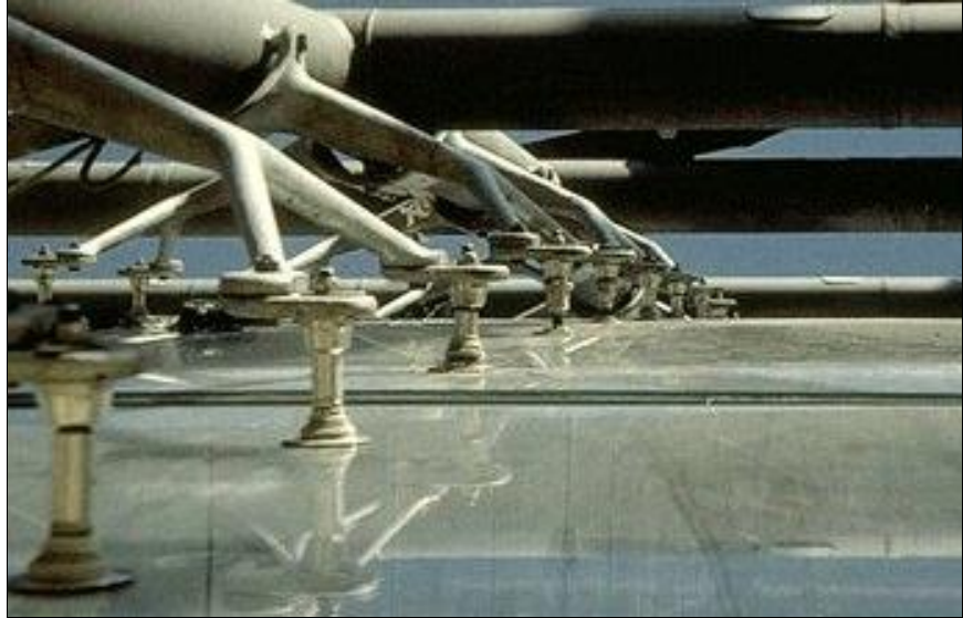
Figure 3 Cast arms and stainless steel point supports
